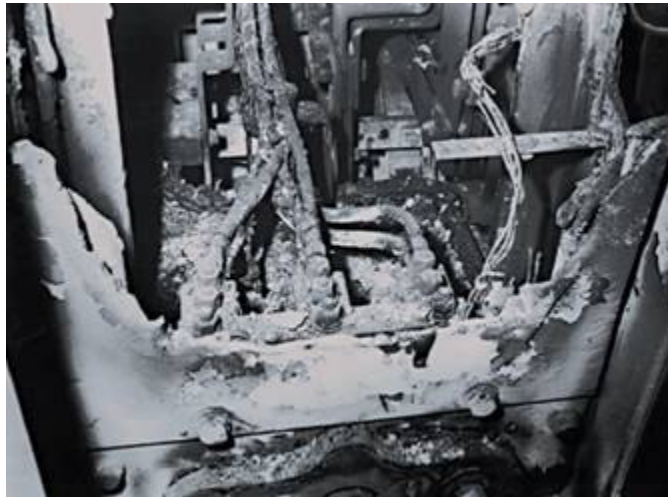
Figure 1.2: Damage from arc-initiated fire in navy shipboard systems [6]
