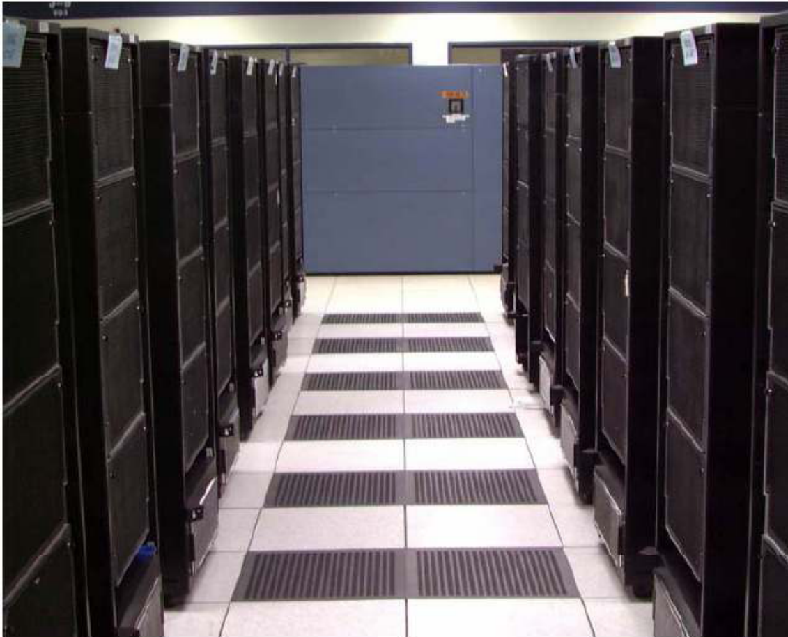
Figure 1.1: Raised floor data center showing racks and perforated tiles [14]
