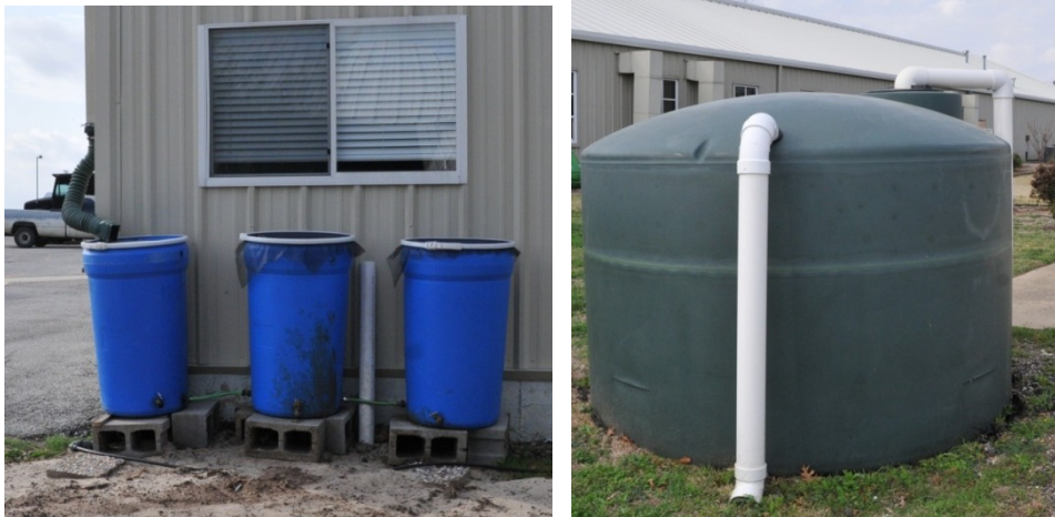
Figure 2.10 Rainwater Collection at Texas Agrilife Research and Extension Center Dallas, TX
