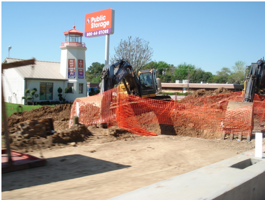
Construction on the North Side of 121 Directly in Front of a Business
