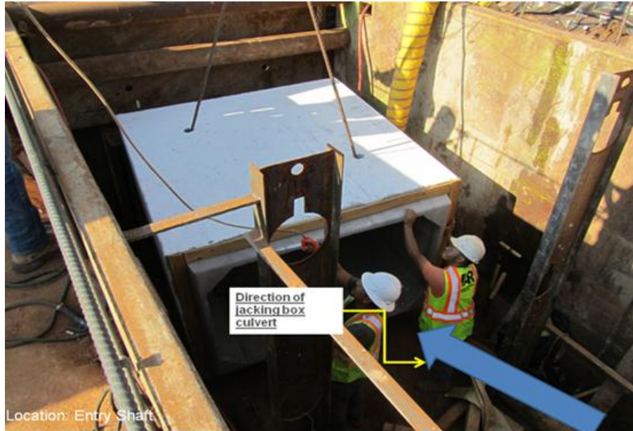
Figure.3.17: Excavator Lowers the Into the Entry Shaft and Two Helpers Guide the Into the Jacking Direction
