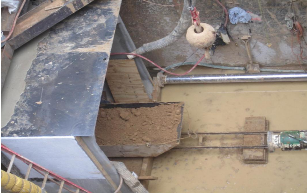
Figure.3.6: Soil Loaded On a Bucket at the Rear End of the Jacking Pit
