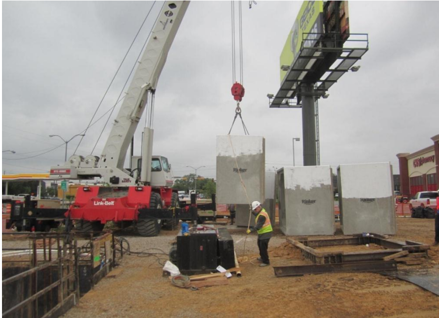
Figure.3.4: A Segment Being Lifted by Mobile Crane from Ground Surface to be Placed in the Entry Shaft
