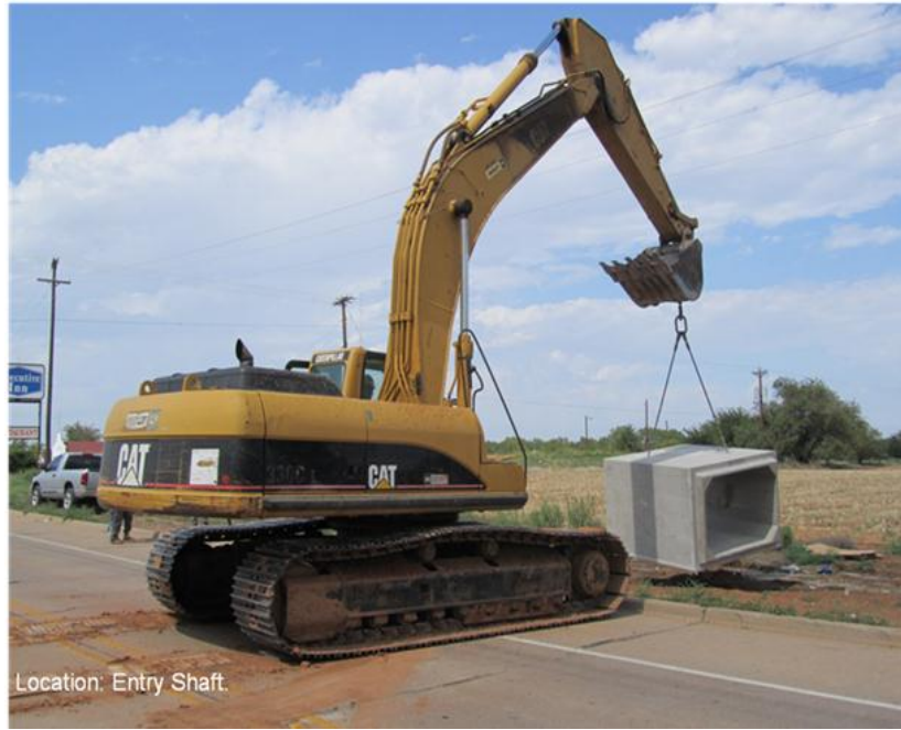
Figure.3.16: Excavator Is Lifting a Culvert and Transporting It to the Entry Shaft
