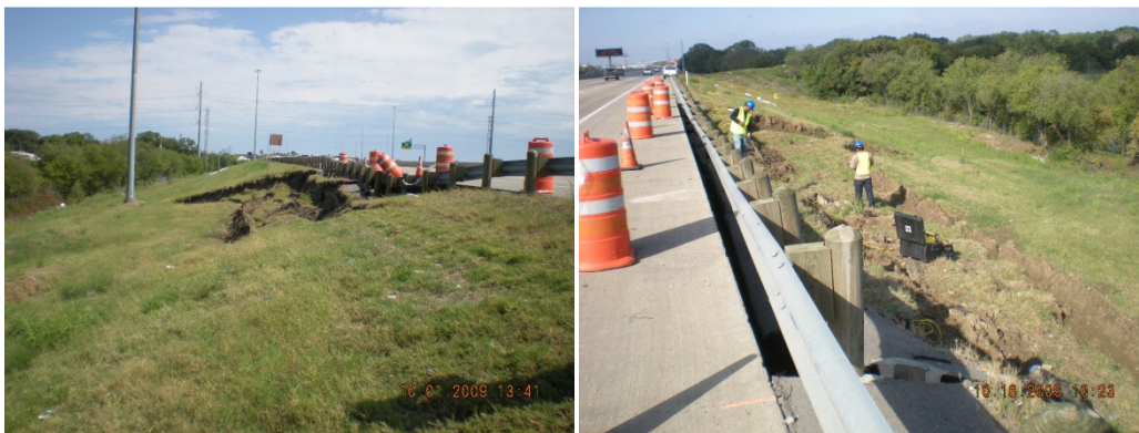
Figure 1.1 Slope failure along I 30 West Bound
