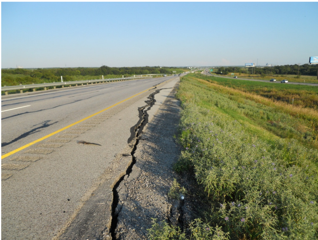
Figure 3.1 Tension cracks along the shoulder
