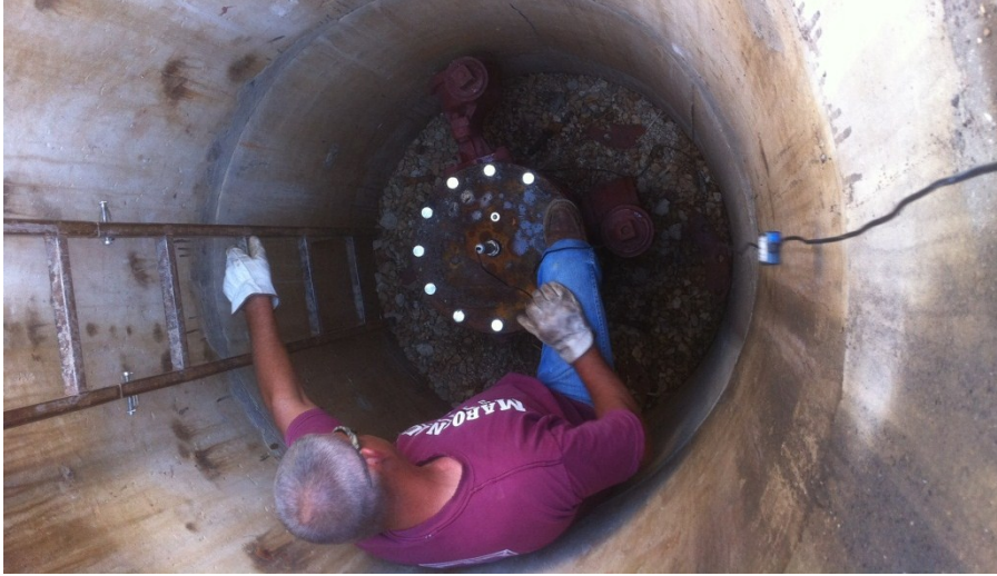
RC Sta. 2087+04 Blow off (Ebenezer Road)
