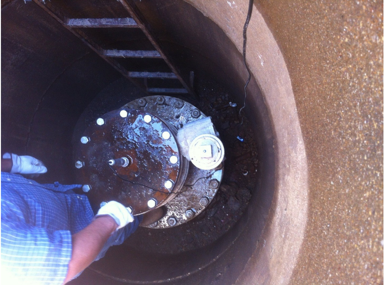
RC 3726+16 Blow-off (Highway 31)
