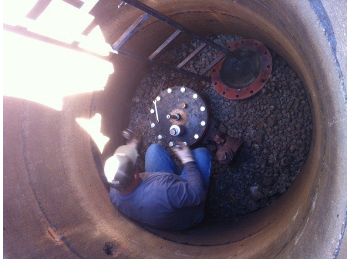
Figure 3: Transducer Connected to Pipeline - Sta. 3873+60
