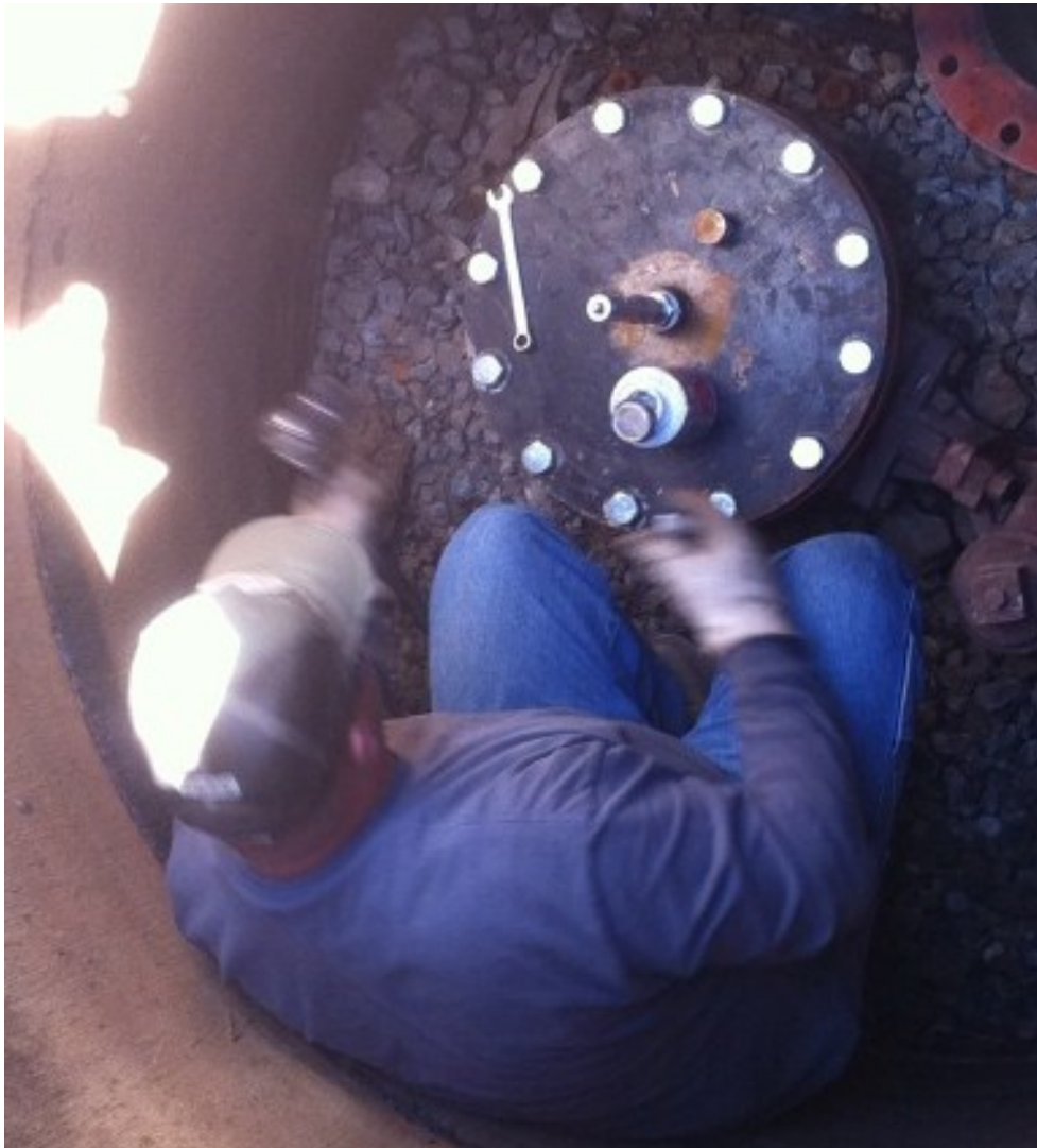
Figure 2.4: Transducer Connected to Pipeline – Cedar Creek Sta. 3873+60
