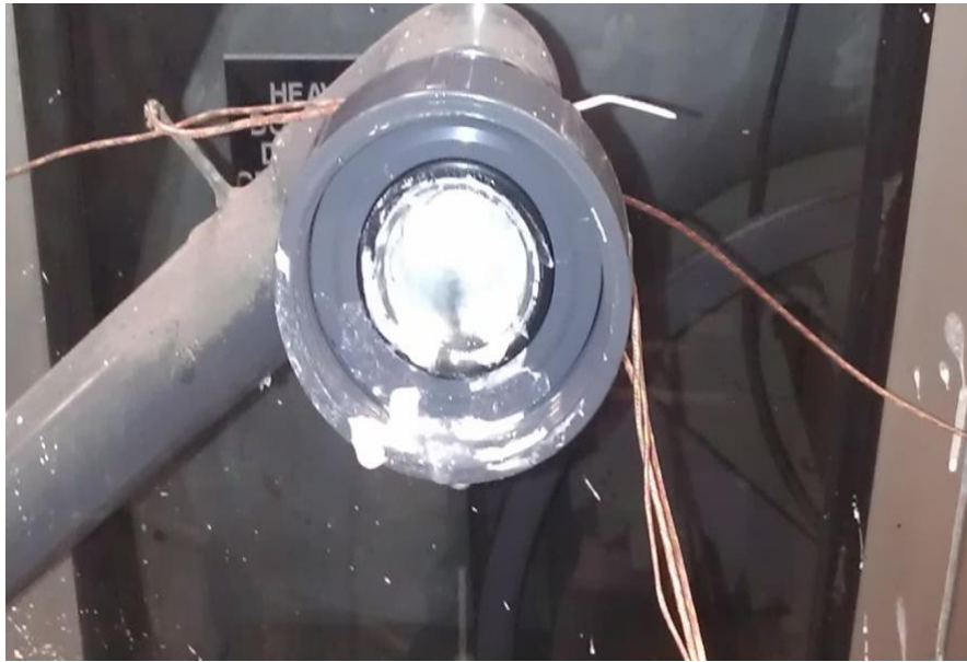
Figure 5.3: Clogged slurry inside the circulating pipes
