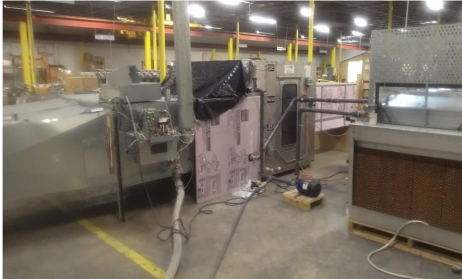
Figure 3.6: Cooling Tower used in Experiment
