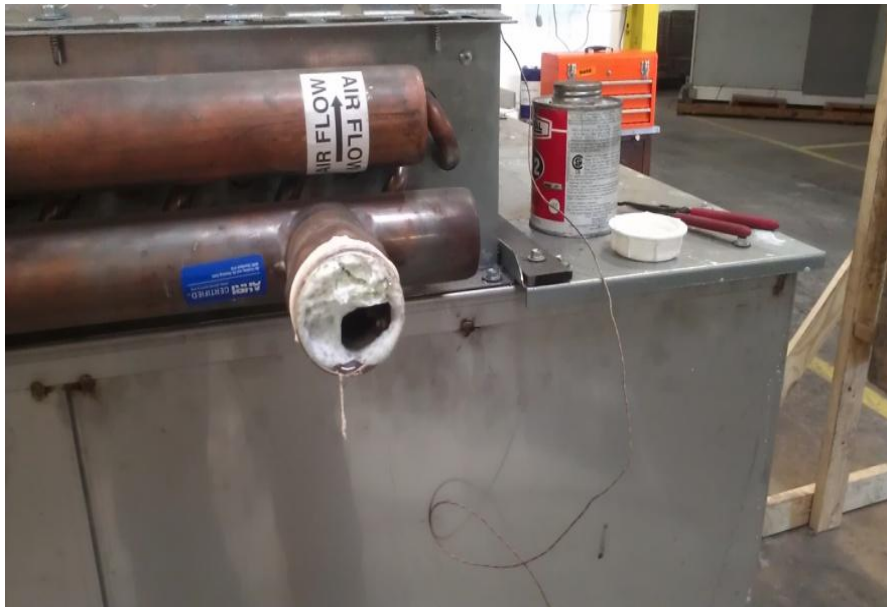
Figure 5.4: Clogging in the pipe at the outlet of cooling Tower
