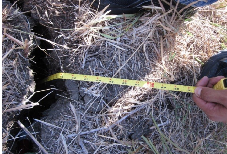
Figure 4.70. 24ft. crack at Joe Pool Dam
