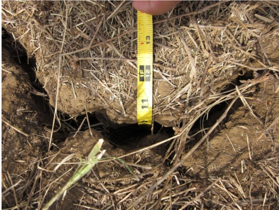
Figure 4.66. Surficial crack 10.5 in depth on control section (Grapevine Dam August 12, 2011)
