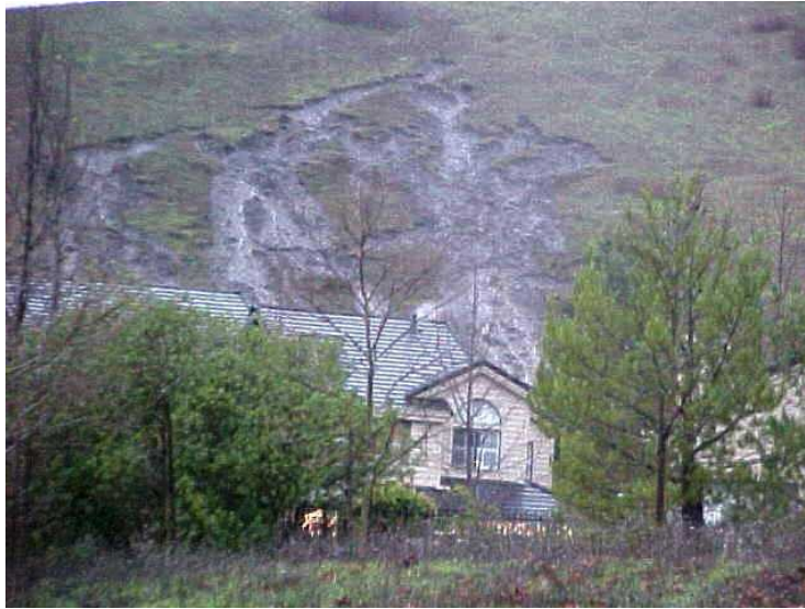
Figure 2.26. One of 60 shallow landslides occurring on December 15, 2002 in Blackhawk, California (Short et al., 2005)
