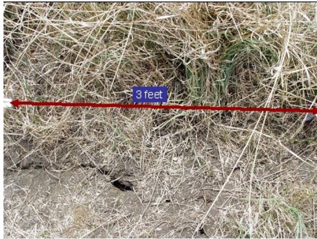
Figure 2.30. Cracking on the slope of Joe Pool dam (Dronamraju, 2008)
