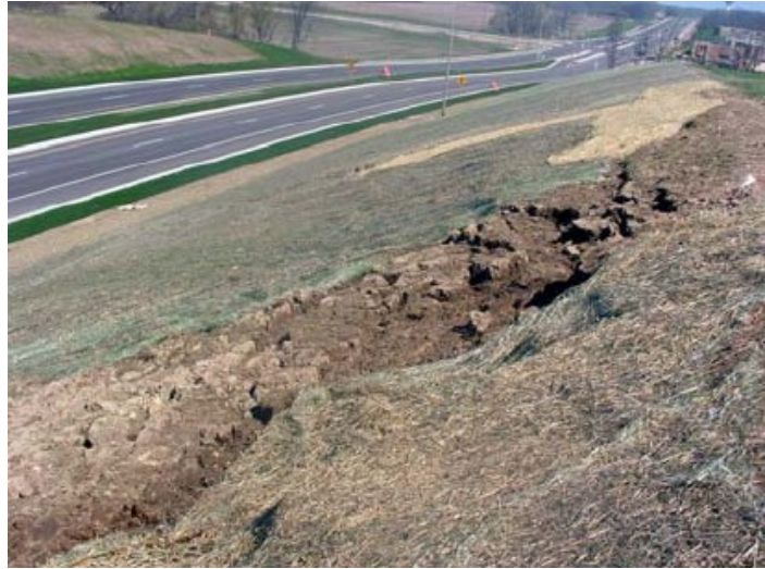
Figure 2.47. Surficial failure on a cut slope along STH-164, Wisconsin (Titi and Helwany, 2007)
