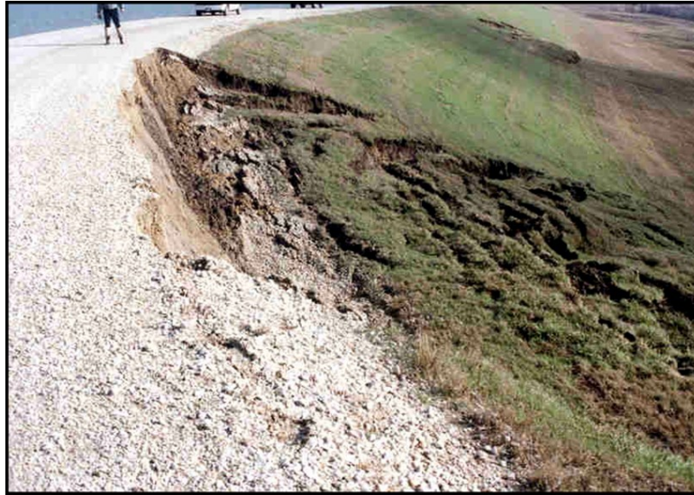
Figure 2.6. Surficial failure at Bardwell Dam (USACE)
