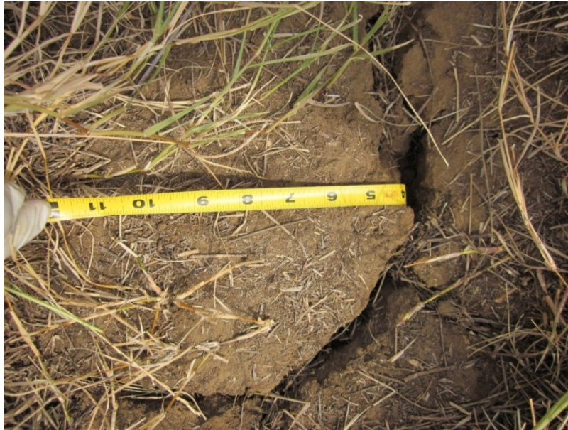
Figure 4.68. Surficial crack 4in depth on compost section (Grapevine Dam August 12, 2011)
