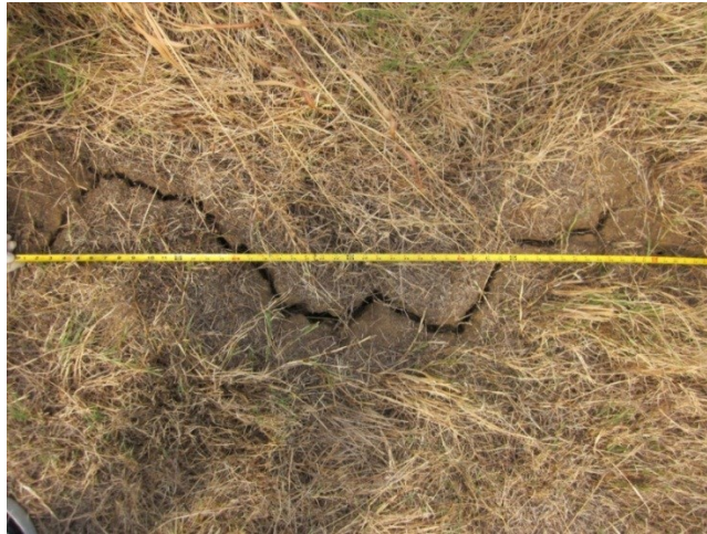
Figure 4.64. Surficial crack 4 ft. length on control section (Grapevine Dam August 12, 2011)
