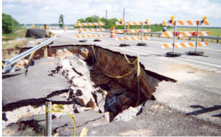
Figure 2.51. Slope Failure at US-71 (Parr, 2007)
