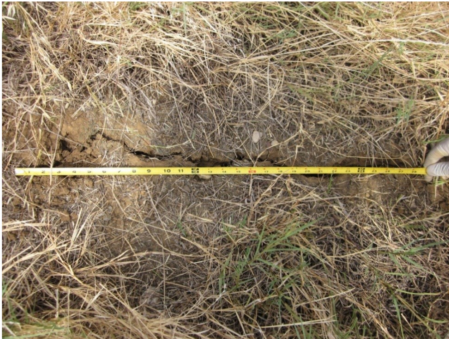
Figure 4.67. Surficial crack 2.3 ft. length on compost treated section (Grapevine Dam August 12, 2011)
