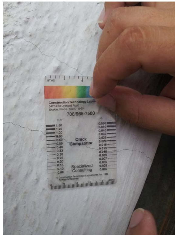
Figure 2.21 Crack at spring line
