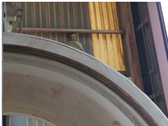
Figure 2.17 Delamination of mortar coating from core
