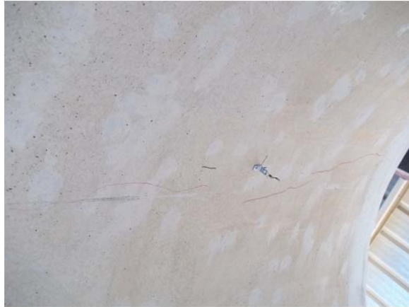
Figure 2.15 0.001 inch crack at crown
