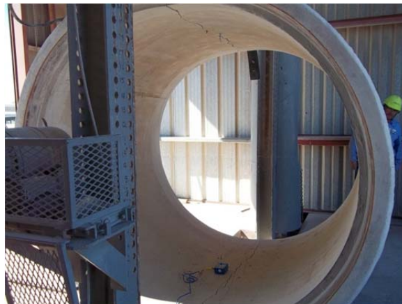
Figure 2.20 Cracks at invert and crown
