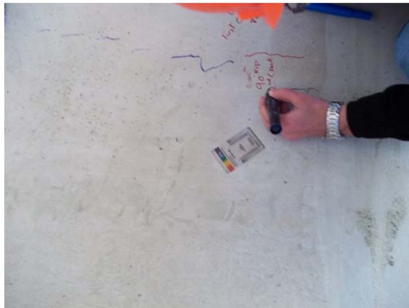
Figure 2.16 0.01 inch crack at invert
