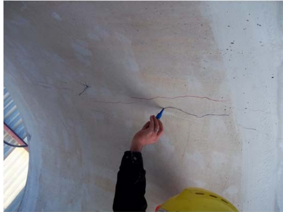
Figure 2.18 0.016 inch crack at crown
