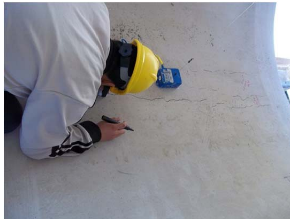
Figure 2.19 0.02 inch crack at invert
