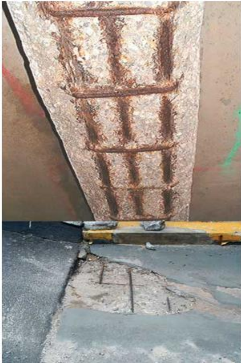
Figure 1.3 Corrosion of reinforcement in reinforced concrete ( www.structuremag.org ).
