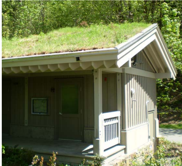
Figure 2.3 A green roof at the Cedar River Watershed outside of Seattle, Washington.
