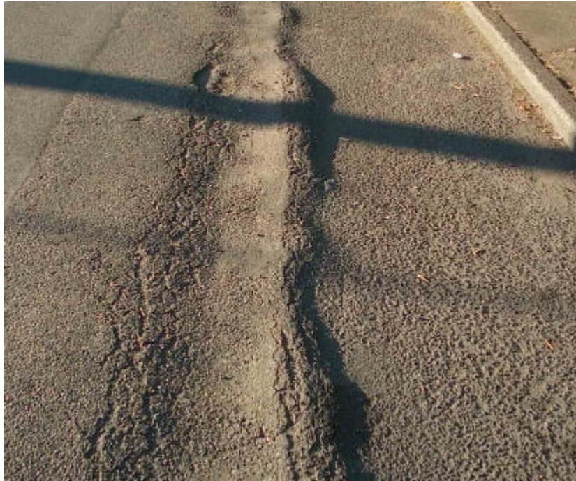
Figure 7.1 Picture showing rutting in a flexible pavement
