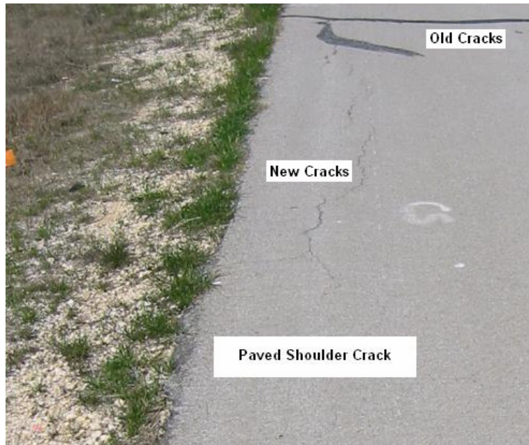
Figure 4.14 Paved shoulder cracks on the Control Plot at Stephenville site
