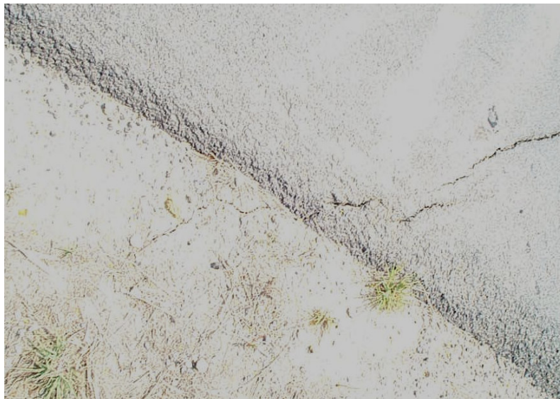
Figure 1.1 Shoulder cracking of SH 108 (Transverse Cracks)
