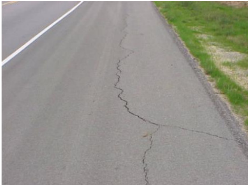
Figure 1.2 Longitudinal and transverse cracks
