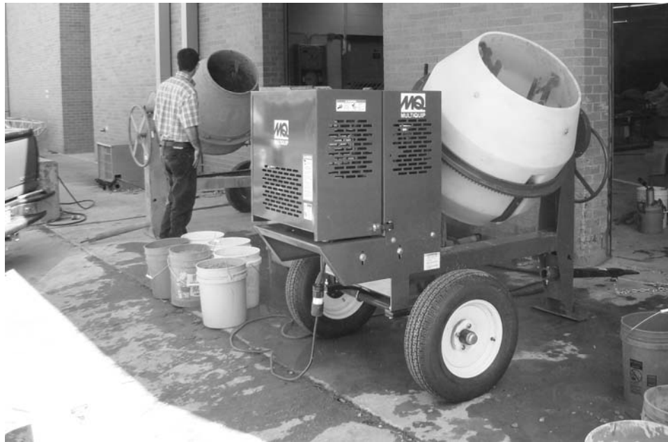
Figure 3-2 Rotary concrete mixers. Two batches were made per mixer for each test
