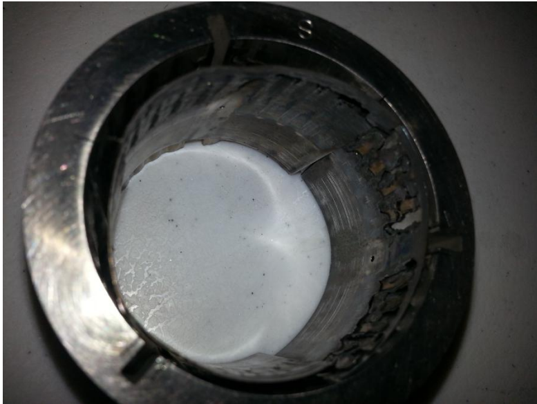
Figure B- 0-3 Front Bearing failure
