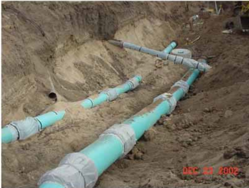
Figure 2.8: Improper Bedding Conditions Leading to Uneven External Pressure on PVC Pipes (Lackey, 2010)
