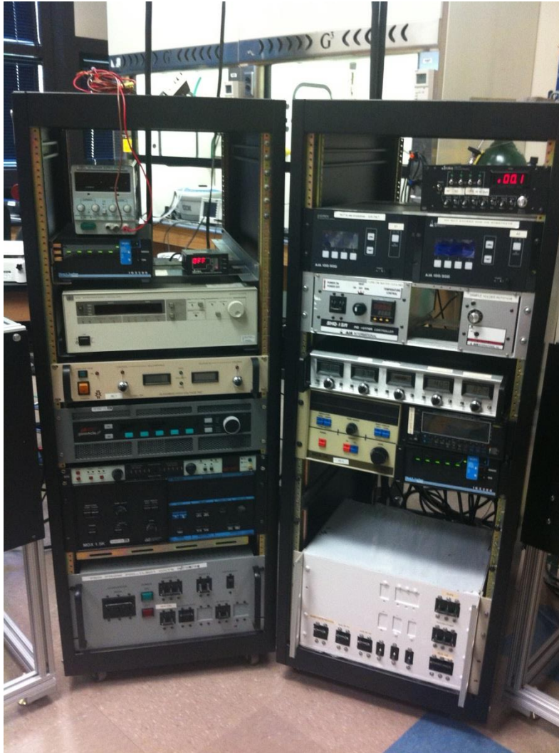
Figure 3-6 Power Supply and Control Panel for PVD Reactive Magnetron Sputtering System in SaNEL
