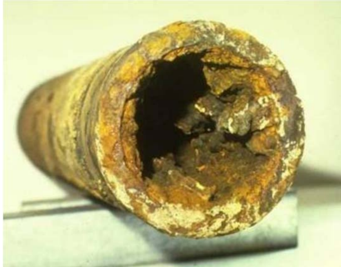
Figure 1.12 - Intensity of Tuberculation Present in Some Cast Iron Water Pipes (Source: 3M Water Infrastructure)
