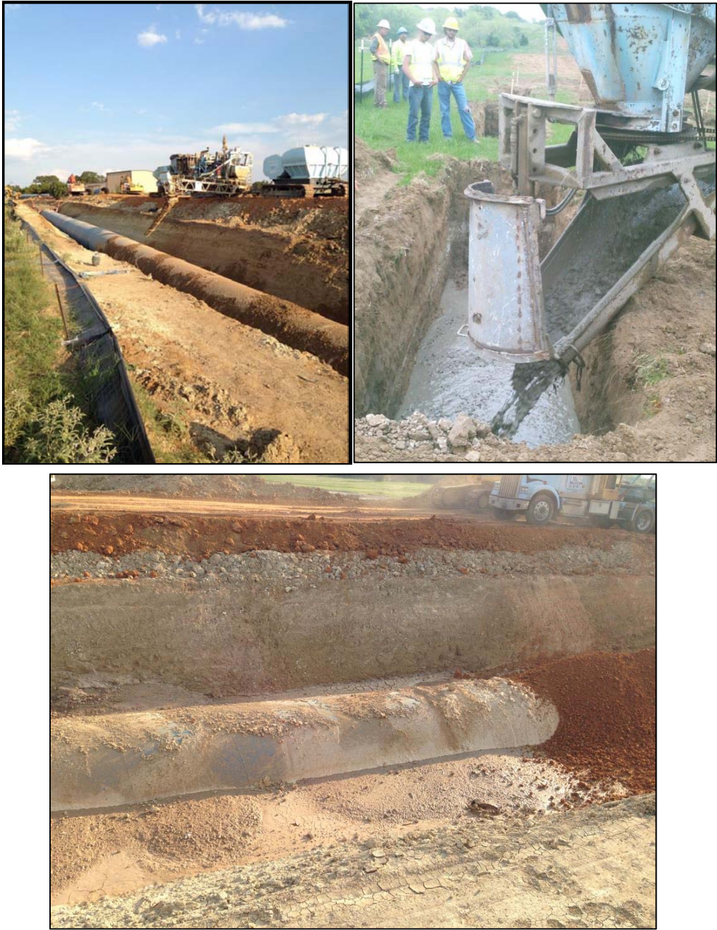
Figure B CLSM Mix Being Poured as Pipeline Bedding Material for IPL Project
