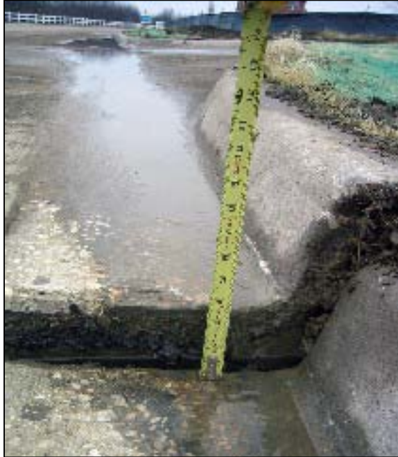
Figure 2.5 Differential vertical movement caused by expansive soil measures 3.5 inches at a pavement joint failure in the Meadow Creek subdivision in Frisco, Texas (Source: Richard J. Hammerberg, P.E, www.cenews.com )
