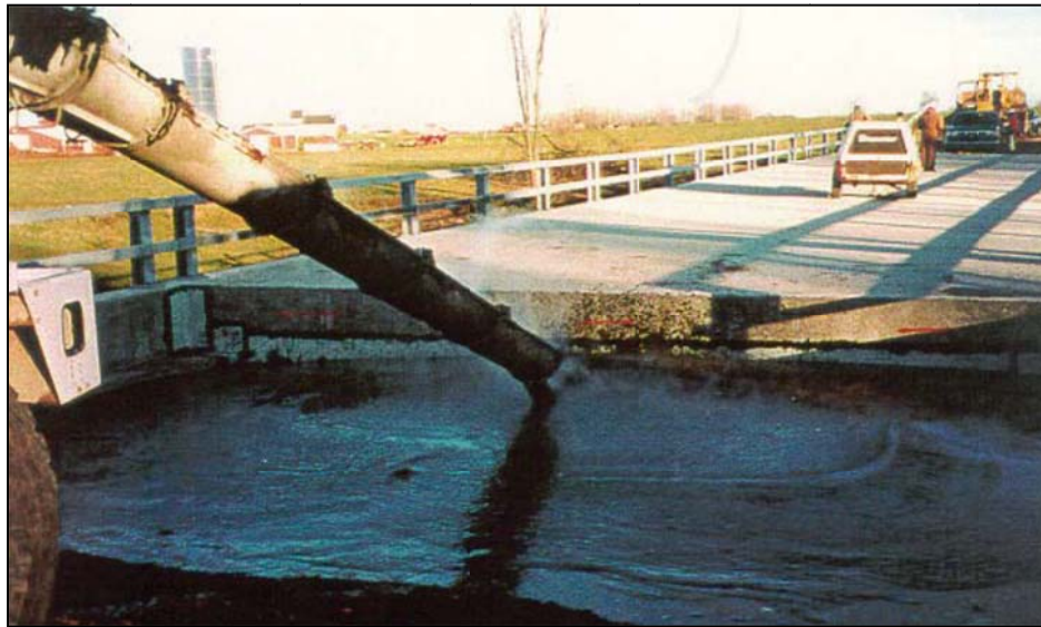
Figure 2.1 CLSM being Used as a Backfill for Bridge Abutment in Wisconsin (Wilson, 1999)
