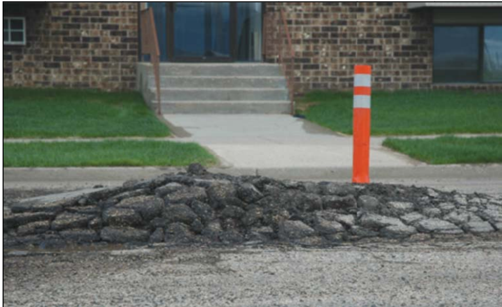
Figure 2.8 Part of Bismarck Street in North Dakota being lifted as a result of frost heave (Manz, 2011)
