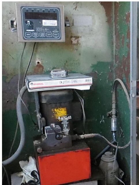
Figure 3-9 Hydraulic Pump, Control Valve, and Pressure Load Cell
