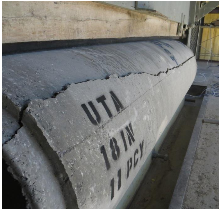
Figure 3-13 Crack Propagation through the Separation Line
