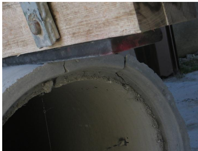
Figure 3-15 Diagonal Crack End
