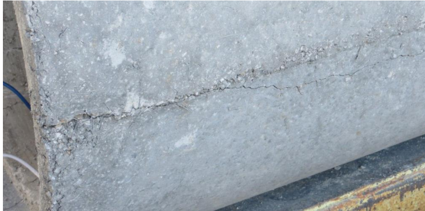
Figure 3-17 Crack Initiation and Propagation through the Separation Line
