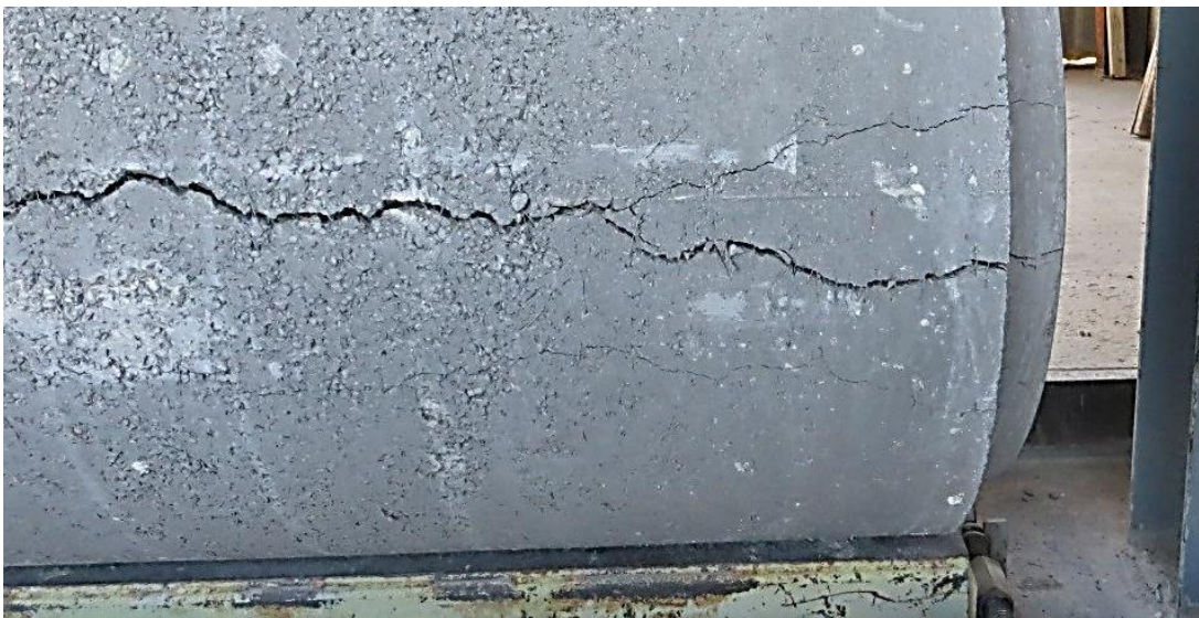
Figure 3-23 Multi Crack Development
