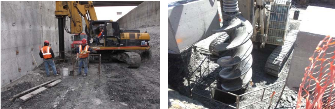
Figure 2-11 Drilling operation for drill shaft walls. (a) drill shaft wall executed in front of a nail wall and (b) protective cage for the operator. (personal pictures archive 2012)
