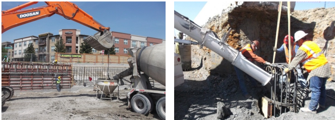
Figure 2-18 (a) Concrete placed in cantilever wall with bucket and (b) drill shaft with hopper (personal archive 2013)
