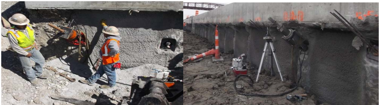
Figure 2-22 Stressing operation for (a) threaded bar tie back wall and (b) low relaxation steel strands
