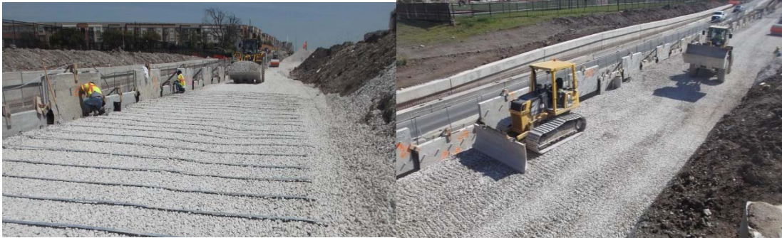
Figures 2.38. Backfilling operation in Wall 4. (a) strip placement over executed lift and (b) loader places backfill over strips to avoid strip damages. (personal pictures archive 2013)
