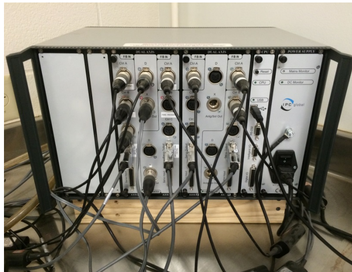
Figure 3.17 Integrated Multi-Axis Control System (IMACS)
