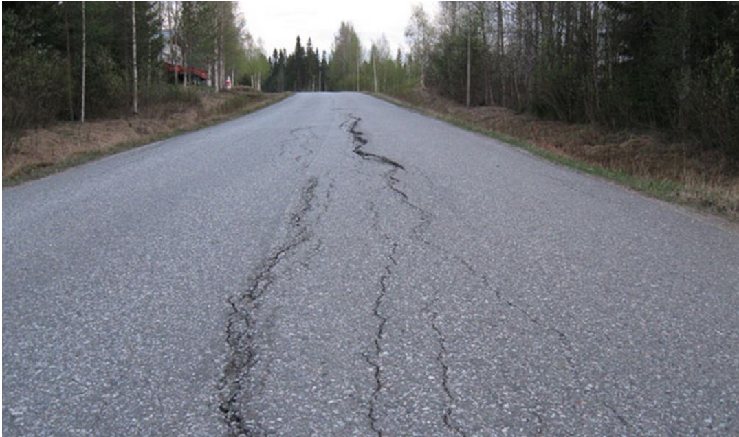
Figure 2.1 Pavement failure due to the swelling of subgrade
