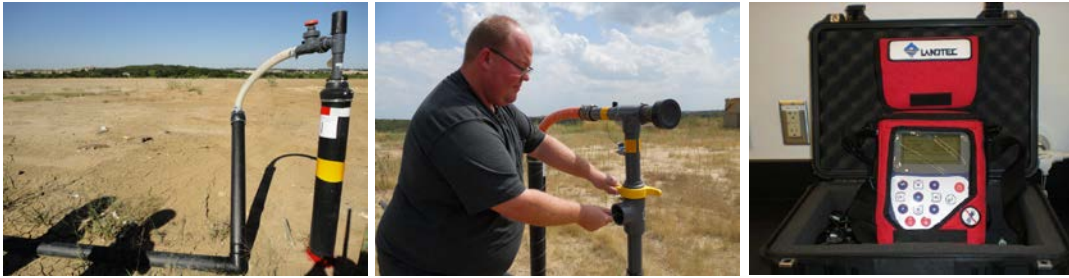
Figure 3.14 Gas Collection Pipe, Flow Measurement and Landtec GEM
