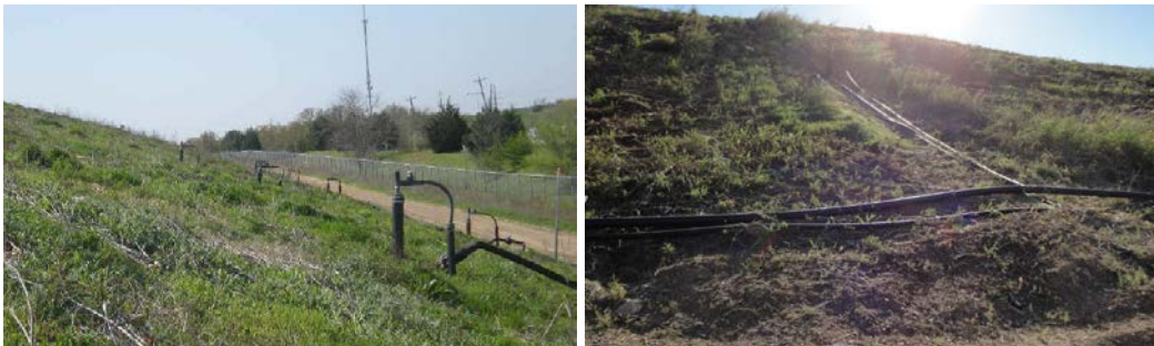
Figure 3.15 Interconnected Leachate Recirculation Pipes in the City of Denton Landfill
