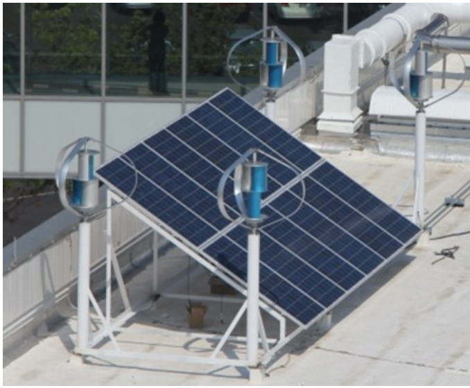
Figure 3.3 UTA MicroGrid Renewable Installation: Photograph of the solar panels, wind turbines, and diesel generator (under solar panels) on the roof of UTA’s Engineering Laboratory Building.
