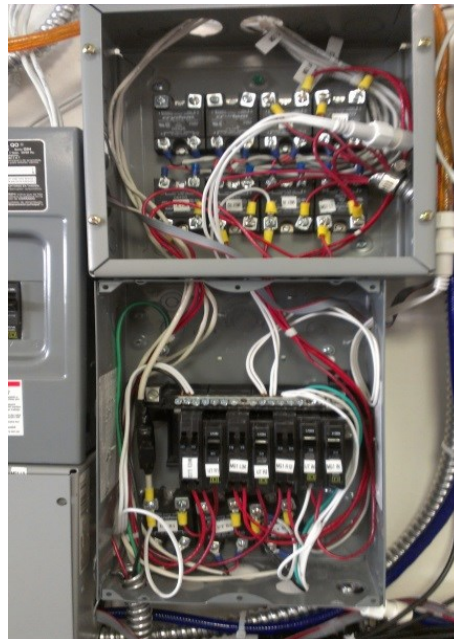
Figure 3.5 UTA MicroGrid 1 Bus Image: Close-up photograph of the NFB and SSR relays used to regulate the flow of power from the legacy electrical grid and MicroGrid 1
