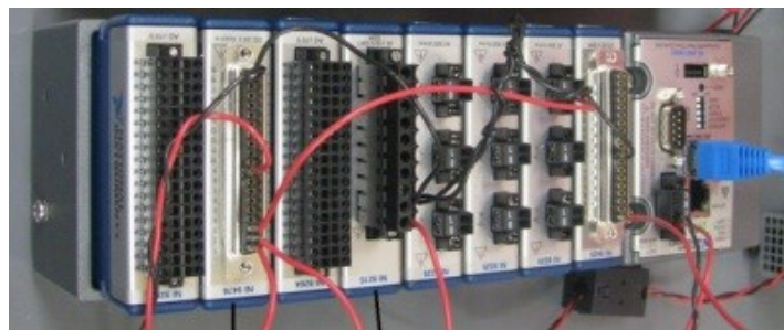
Figure 3.8 National Instruments CompactRIO data acquisition and digital control system.
