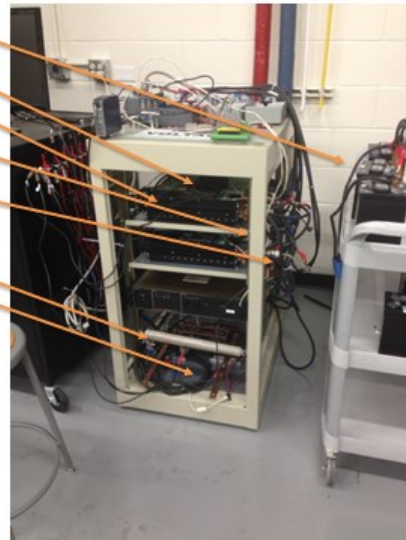
Figure 3.11 COTS HESM Physical Setup: Active Hybrid Energy Storage Control (middle), Monitoring Setup (left), Battery Bank (right)
