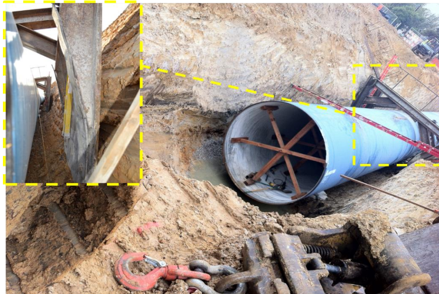
Figure 1-2 Steel trench shield to protect the trench walls from collapsing while excavating
