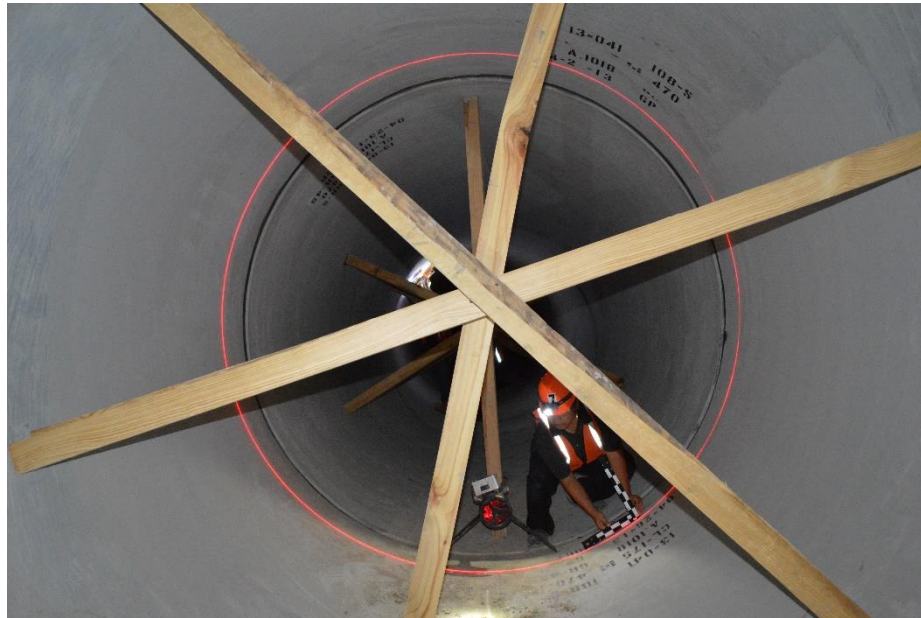
Figure 2-18 Laser photo profile method at end of pipe joint number 1066 at placement
