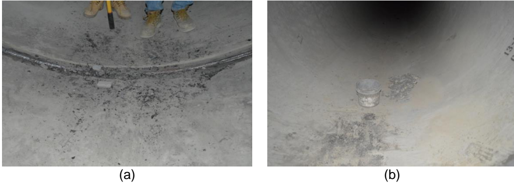
Figure 2-26 Debris within pipeline (a) welding joint debris (b) installation debris
