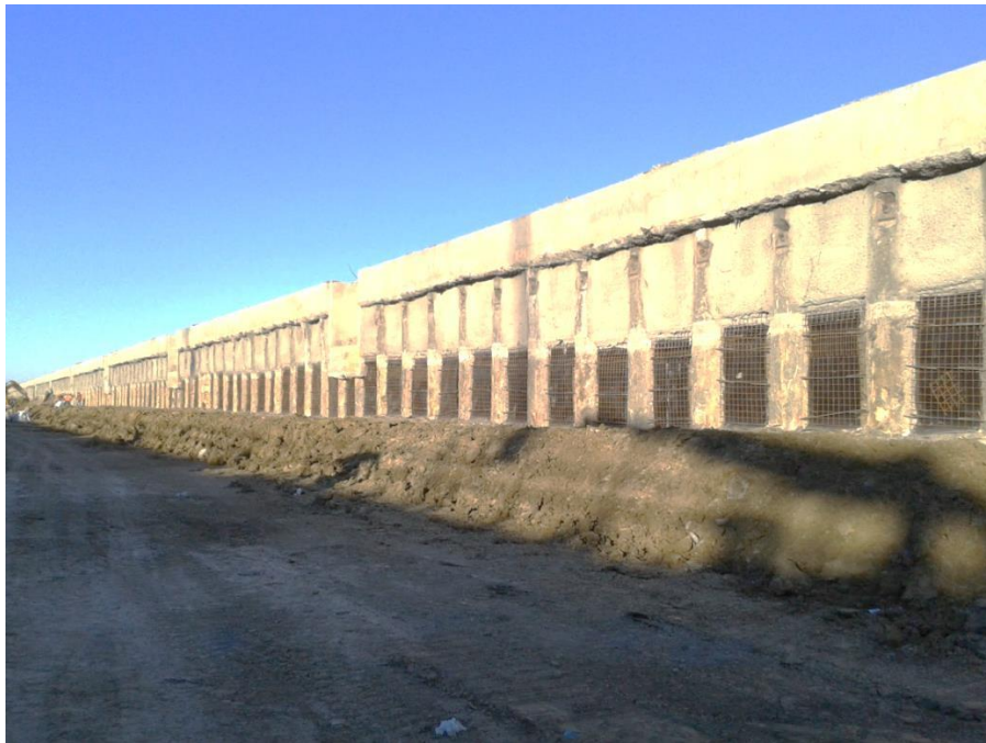
Figure 1.2 A closer look at retaining walls of the "IH-635 Managed Lanes Project."
