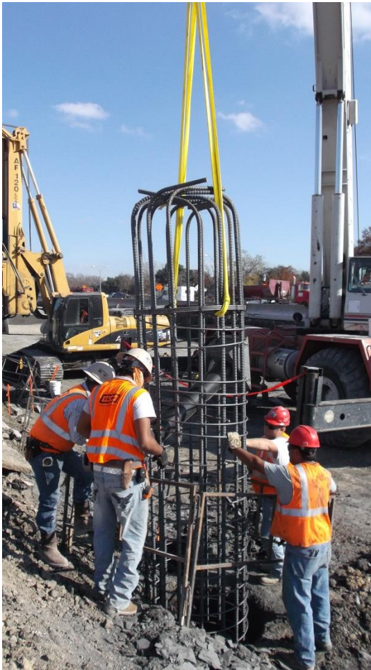
Figure 2.8 Reinforcing steel being installed in the drilled shaft (Personal file, December 3rd, 2012).
