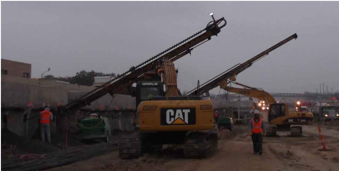
Figure A. 6 Comparison on the width of platform needed by both pieces of equipment (Personal file, January 8 th , 2014)
