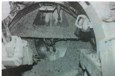
Figure 1-20 Work Face Protection by Means of Plate Flap Pressed by Hydraulic Jack
