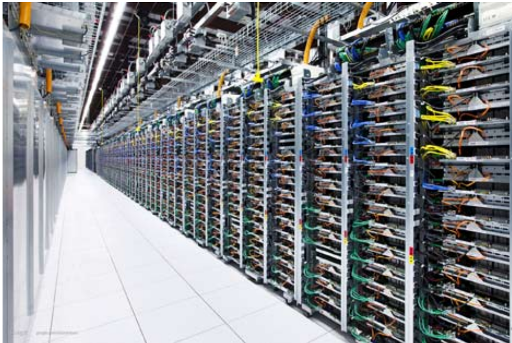
Figure 1-1: The interior of an air-cooled data center
