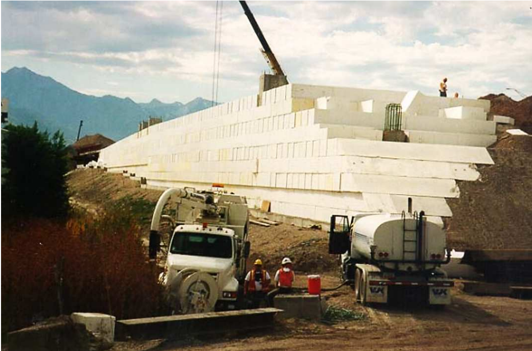
Figure 2.31 Typical geofoam embankment construction on the I-15 reconstruction project in Salt Lake City, Utah (Bartlett et al., 2012)
