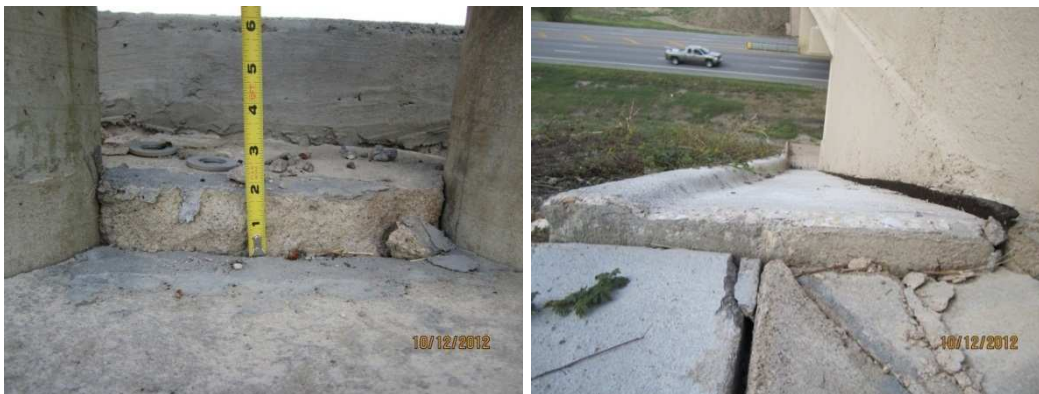
Figure 5.2 Differential settlements occurred in a few months after opening to the traffic
