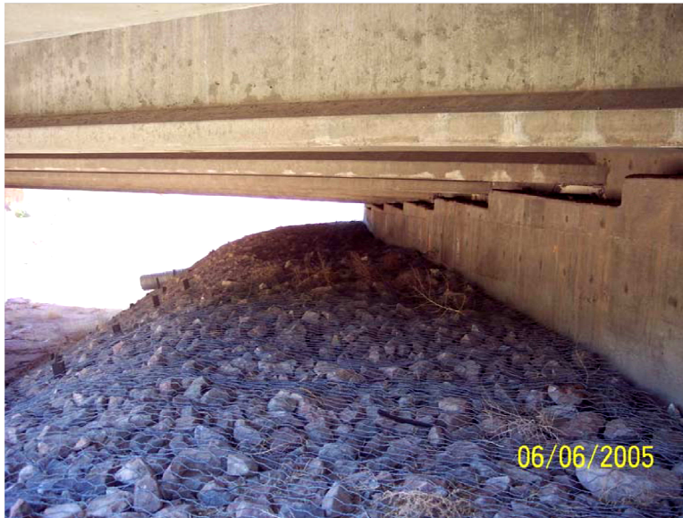
Figure 2.26 Rip-rap system used for erosion control (Lenke, 2006)
