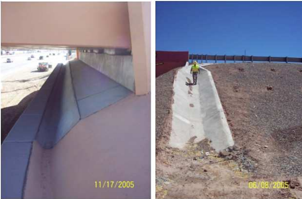
Figure 2.27 Concrete slope protection and drainage channel (Lenke, 2006)
