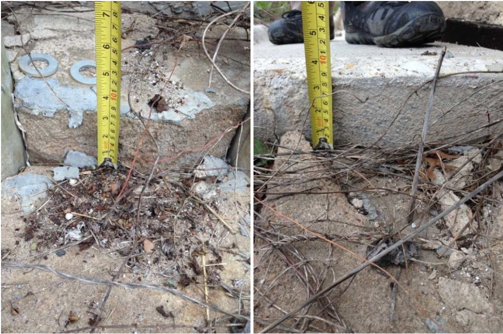
Figure 5.3 Differential settlement occurred in November 2013
