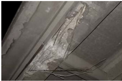
Figure 2-1 Damaged concrete girder (Image Courtesy: TXDOT)
