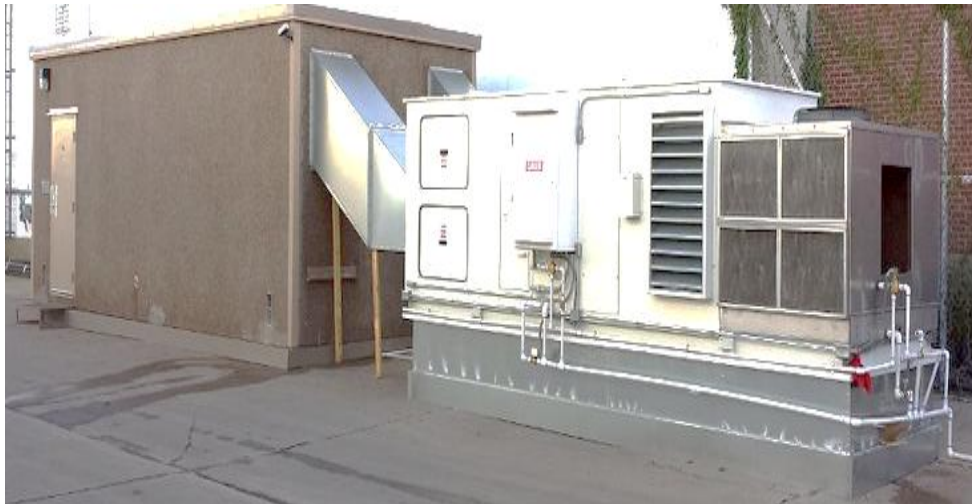
Figure 4.1- Actual IT pod and the cooling system
