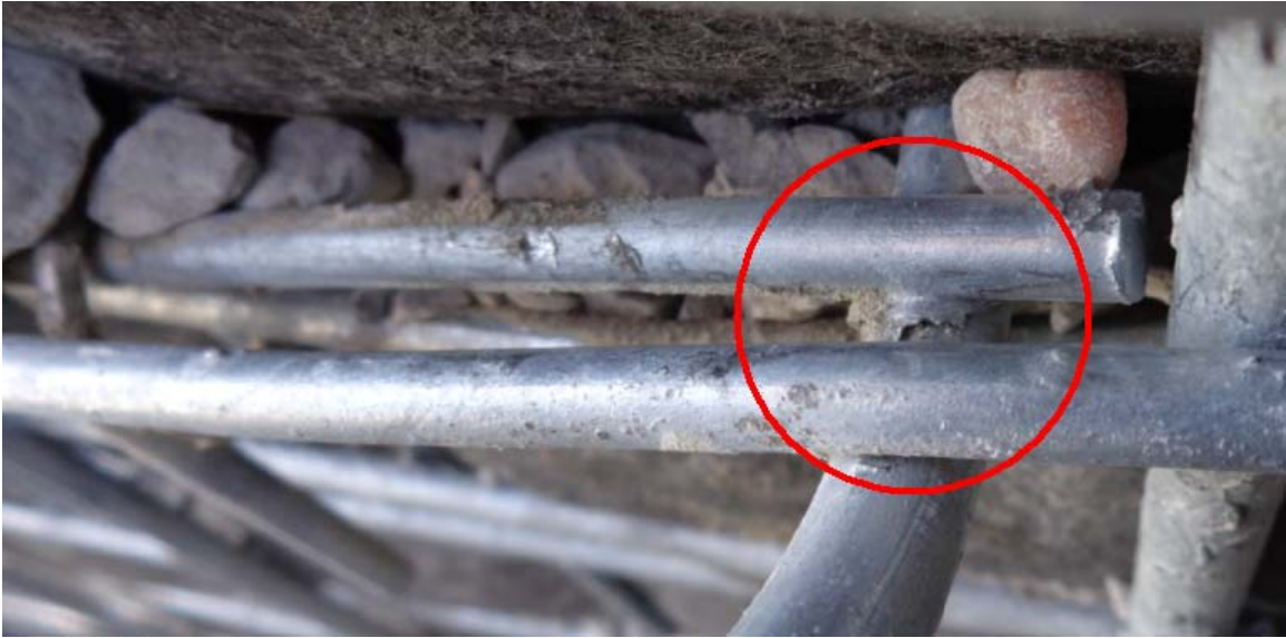
Figure 3-31 Crack at Weld at 100mm Displacement
