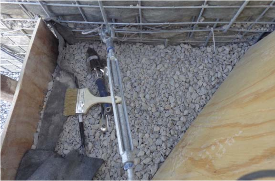
Figure 3-34 Isolated Top-Outside turnbuckle
