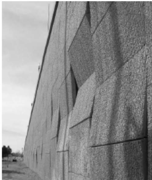
Figure 1-5 Buckling of wall panels in 2-Stage MSE wall (Gerber 2011)
