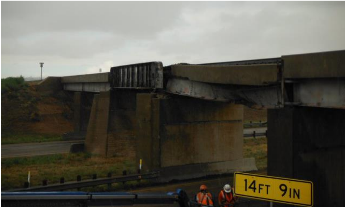
Figure 1 - Damage from Impact
