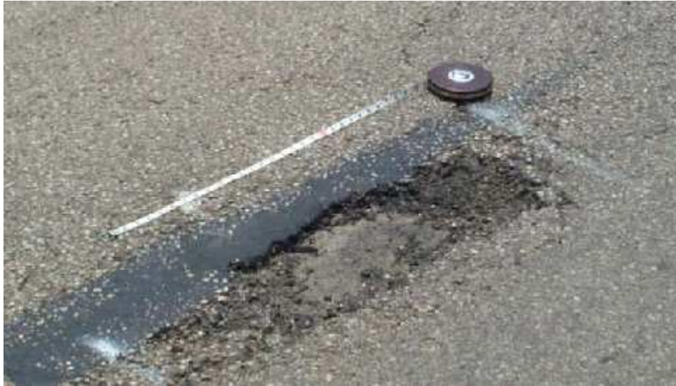
Figure 3-5 Pot Hole in Wheel Path of the Second 0.1 mile Section along Pearce Lane
