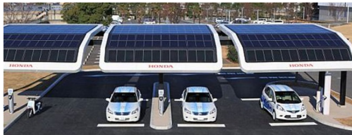
Figure 1-10 Public charging station
