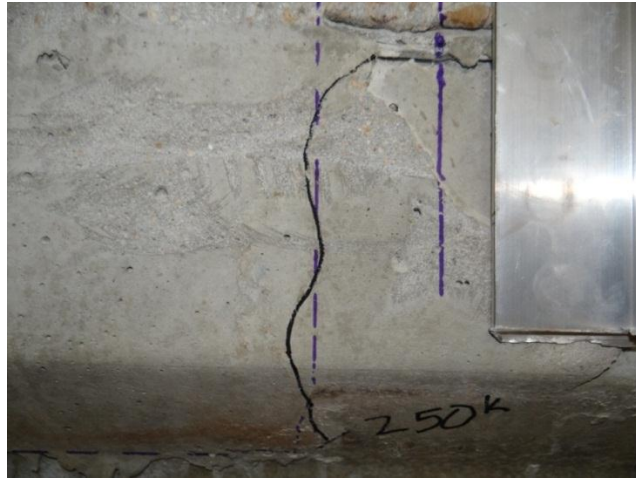
Figure 5-62 Interface cracks at the breakout
