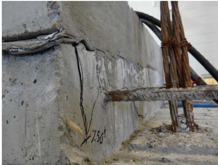
Figure 5-51 Cracking of concrete at East-end
