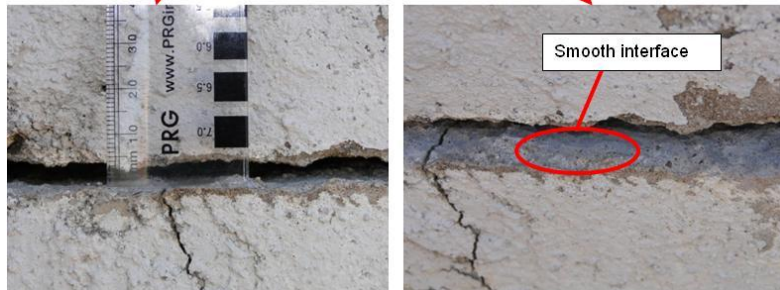
(b) Crack width
