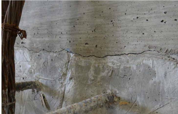
Figure 5-49 Cracking at the interface on beam end
