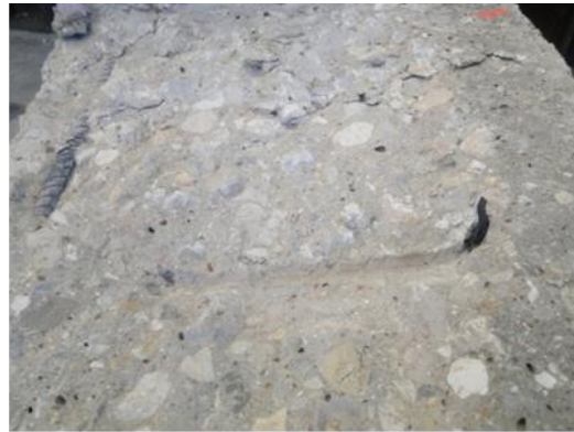
CIP slab failure plane
