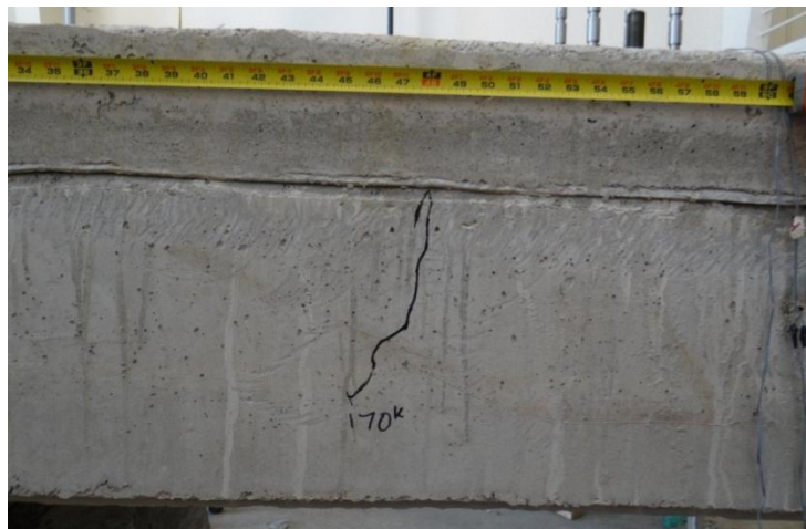
Figure 5-38 Vertical cracks close to beam ends (South-West side)
