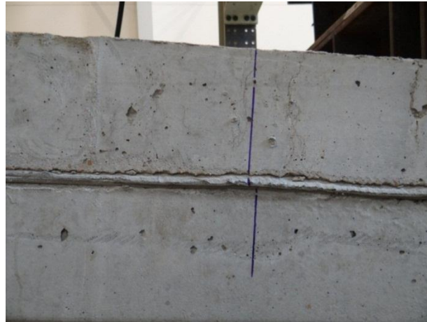
Figure 5-67 Interface slip at failure
