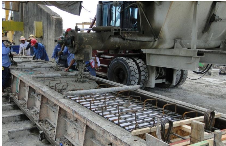
Figure 4-46 Casting of the top part of the box beam with horizontal shear reinforcement
