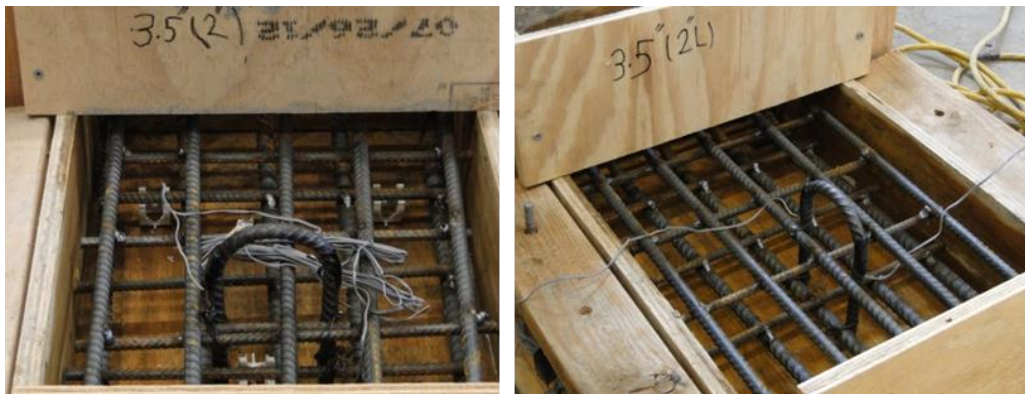
Figure 4-22 3.5-in. wide horizontal shear reinforcement with 2-in. embedment (180° bend) placed in the (a) transverse and (b) longitudinal direction
