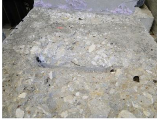
CIP slab failure plane
