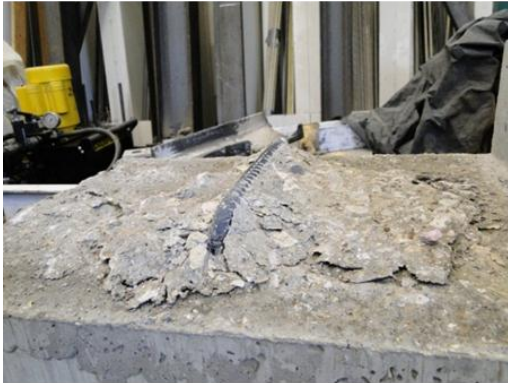
Precast failure plane
