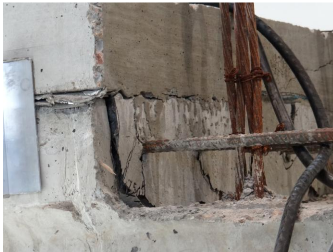
Figure 5-54 Fracture of concrete at East-end (close view)
