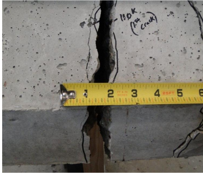
Figure 5-26 Crack width at failure
