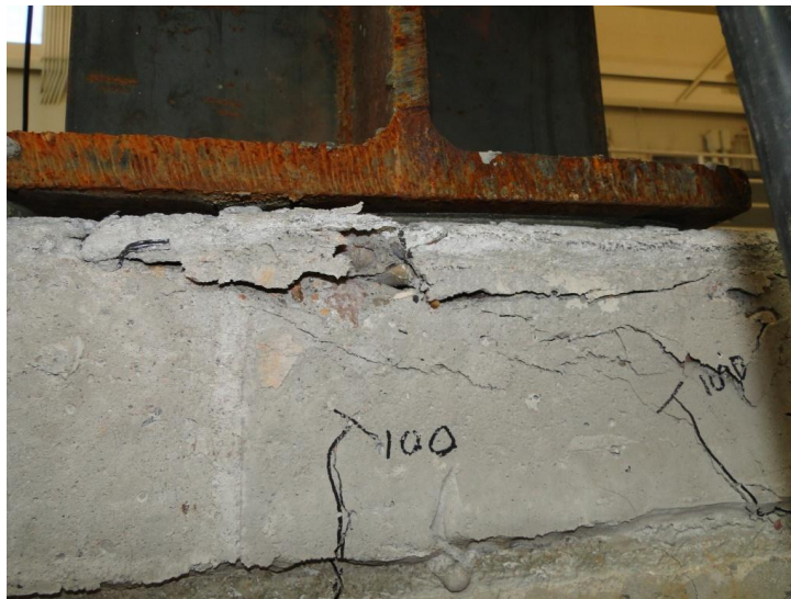
Figure 5-13 Crushing of concrete at loading point
