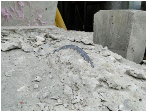
Precast failure plane
