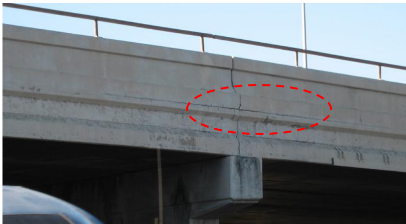
Figure 1-3 Interface cracks on Riverside Dr. Underpass at I-35
