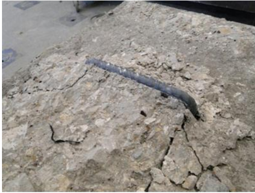
Precast failure plane
