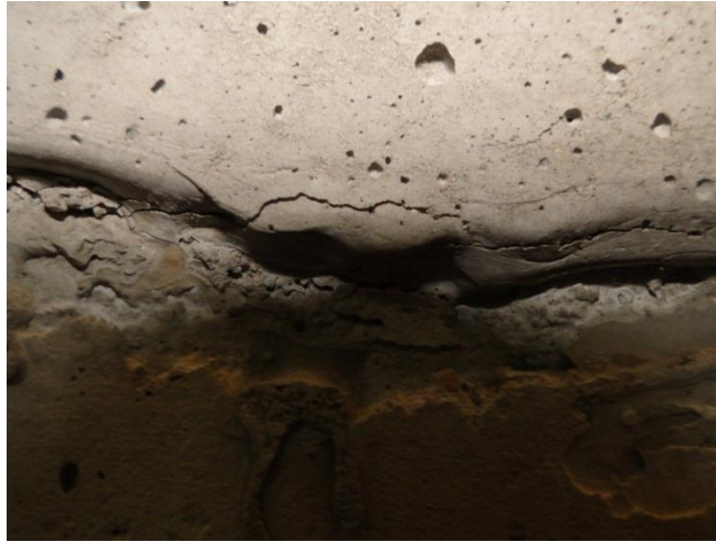
Figure 5-20. Horizontal crack at the interface
