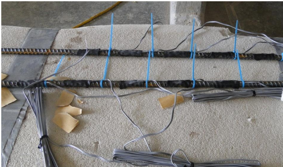
Figure 4-40 Strain gauges on longitudinal reinforcement
