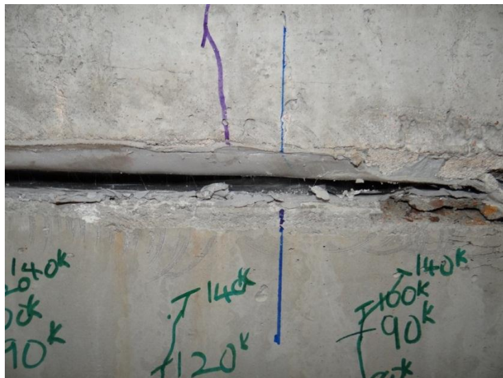
Figure 5-35 Separation of the interface at failure
