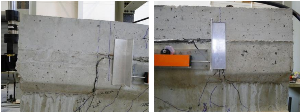
Figure 5-68 Cracks at the interface of the CIP slab and blockout
