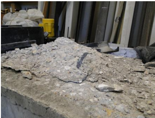
Precast failure plane
