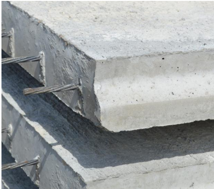
Figure 3-20 Surface roughness on precast panels
