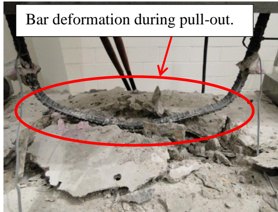
Figure 5-10 Fracture of concrete during pullout
