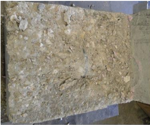
Precast failure plane
