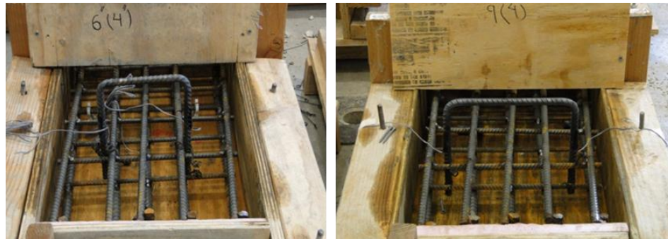
Figure 4-24 (a) 6-in. and (b) 9-in. wide horizontal shear reinforcement with 4-in. embedment (90° bend)
