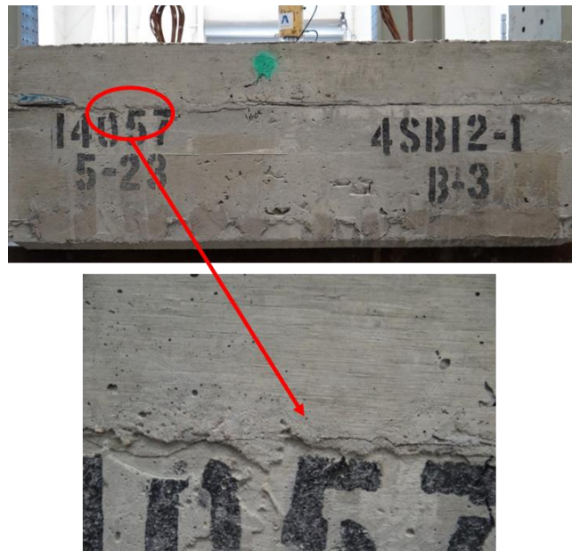
Figure 5-42 Interface cracks at beam ends
