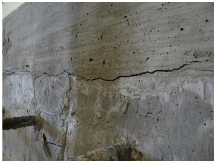
Figure 5-52 Cracking at the interface at beam end
