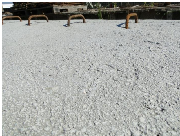
Figure 4-86 Surface finish on slab beam having conventional concrete
