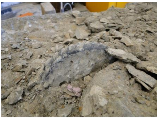
Precast failure plane
