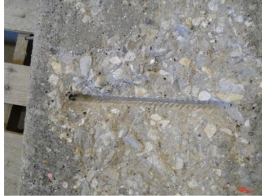
CIP slab failure plane
