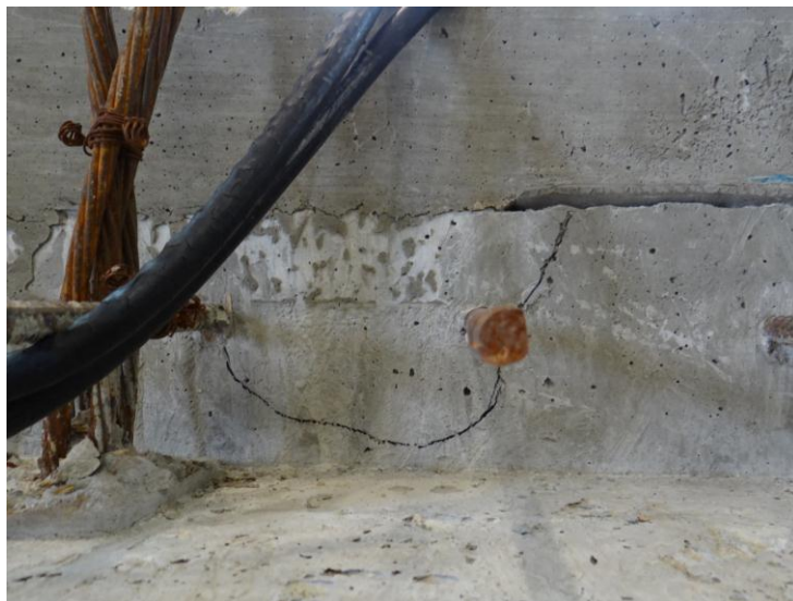
Figure 5-50 Fracture of concrete at beam end
