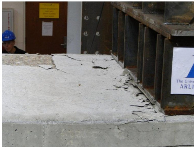
Figure 5-16 Crushing of concrete at the top of the beam at failure
