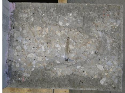
CIP slab failure plane
