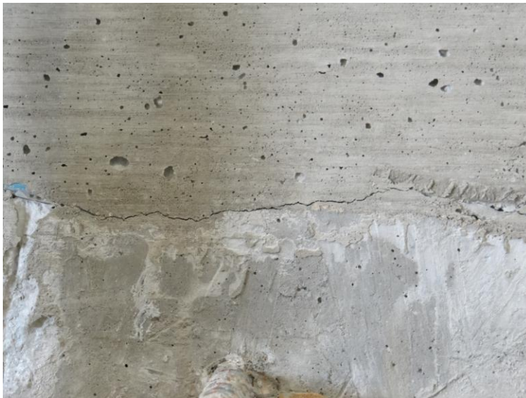
Figure 5-48 Cracks form at the interface
