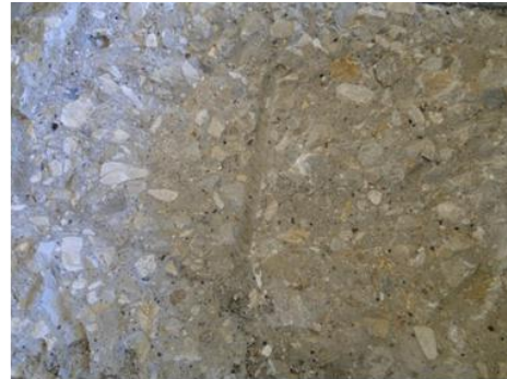
CIP slab failure plane
