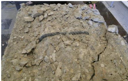
Precast failure plane
