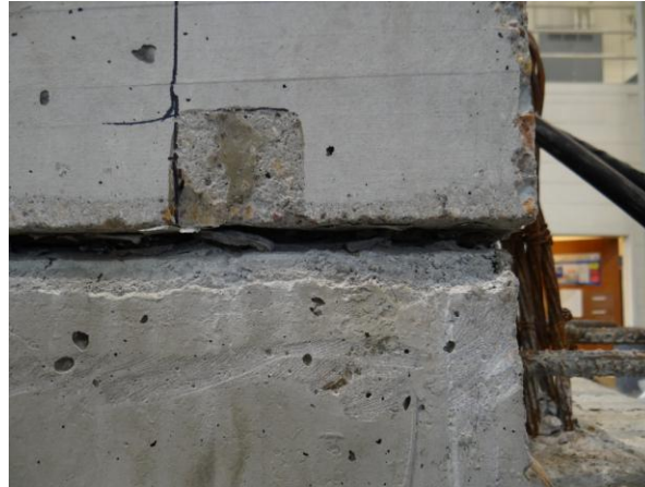
Figure 5-57 Interface slip at failure
