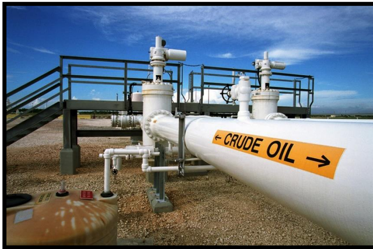
Figure 17 - Crude oil Pipeline
