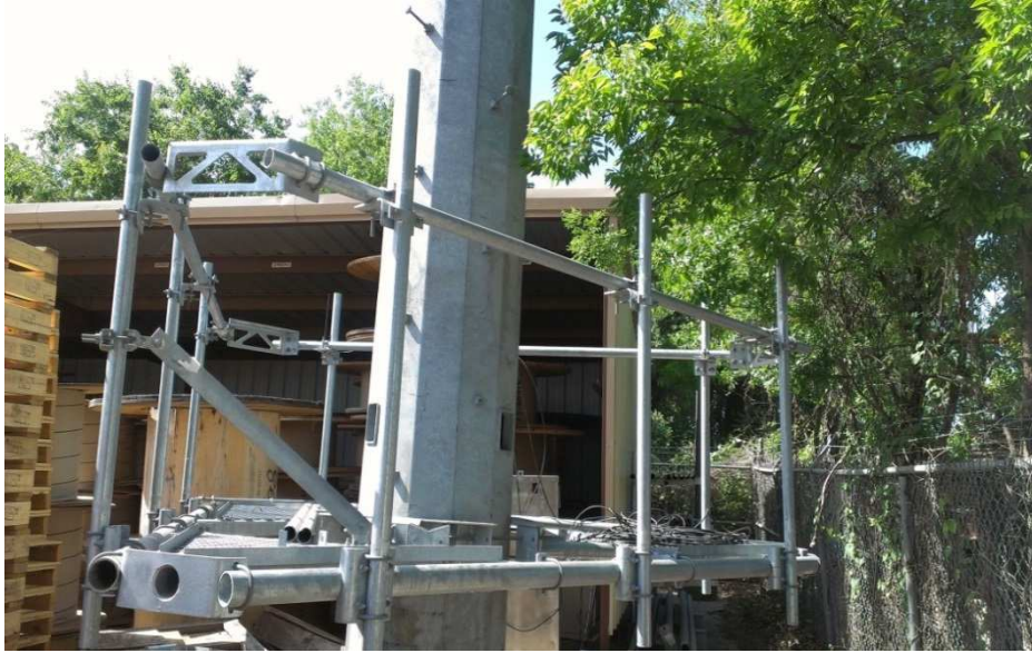
Figure 1.9 Antenna mount carrying three antenna units
