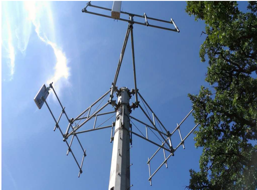
Figure 1.8 Antenna mount carrying four antenna units
