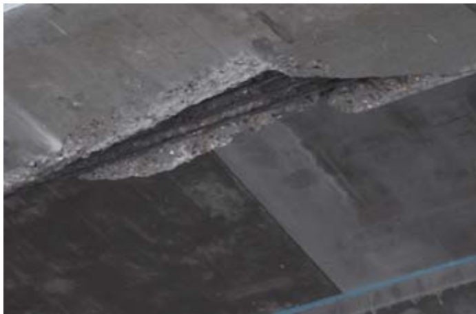
Figure 3-10 Strands Bottom Row Exposed
