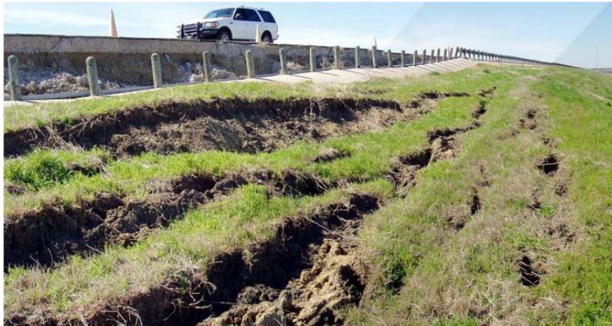
Figure 2-19 Surficial slope failures triggered due to desiccation cracks in Joe Pool dam (McCleskey et al., 2008)
