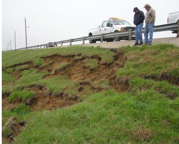
Figure 2-20. Surficial slope failures triggered due to desiccation cracks in Grapevine dam (McCleskey et al., 2008)
