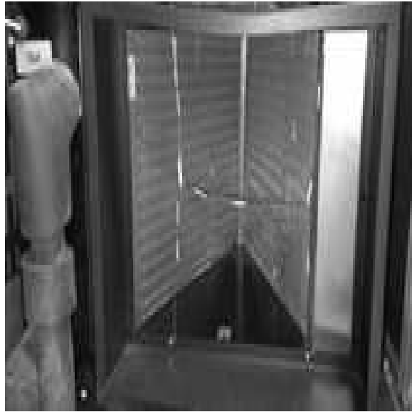
Figure 2.5. Rear view of Heat Exchanger.
