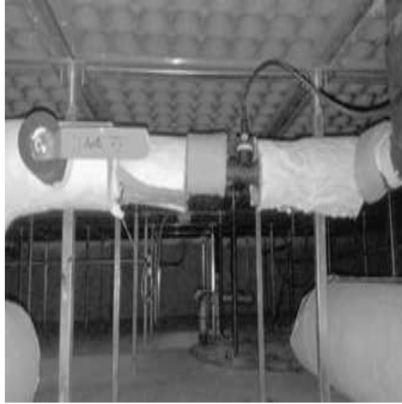
Figure 2.7. Location of vortex flow meter on the supply pipe of heat exchanger.
