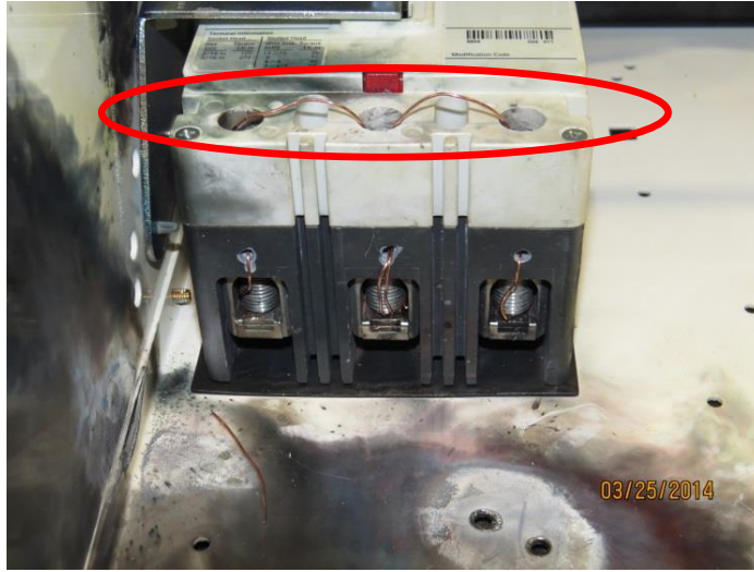
Figure 4- 40 HCB configuration on switchgear
