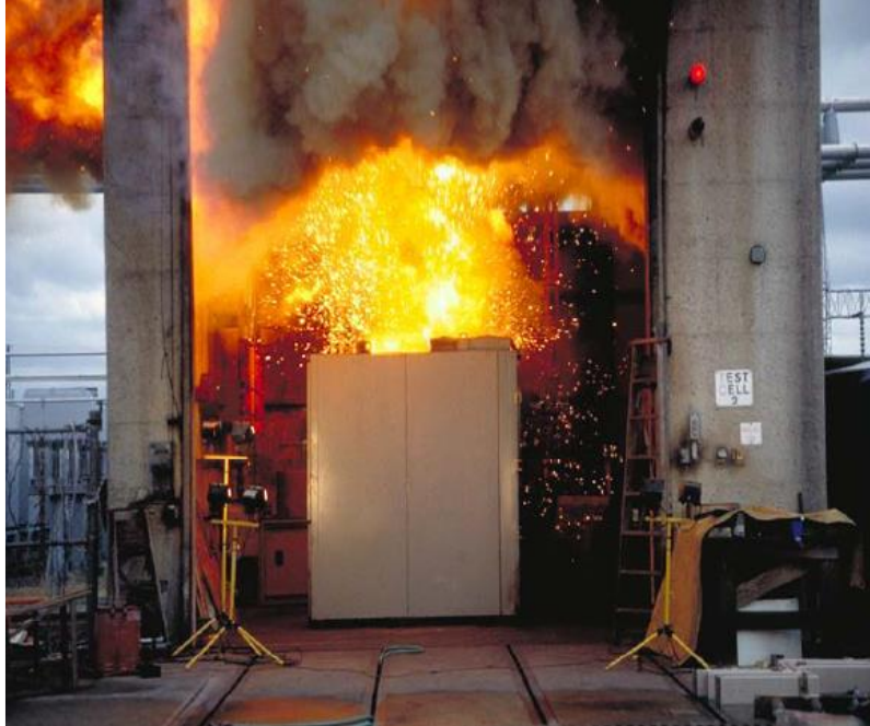
Figure 2- 2 Destructive arc blast in test cell [13]
