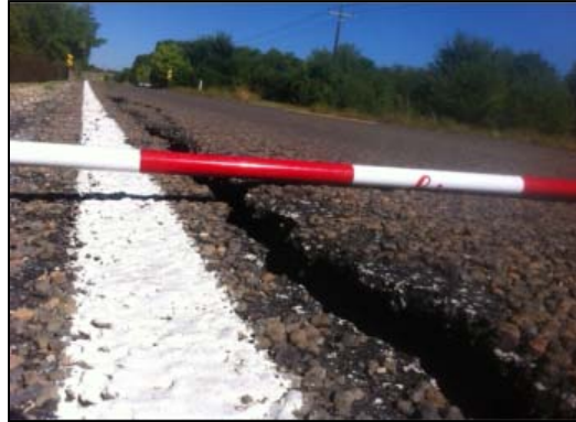
Figure 4. 31: Observed edge drop
