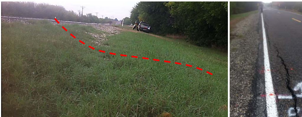
Figure 4. 32: Shallow sliding and top crack in the pavement
