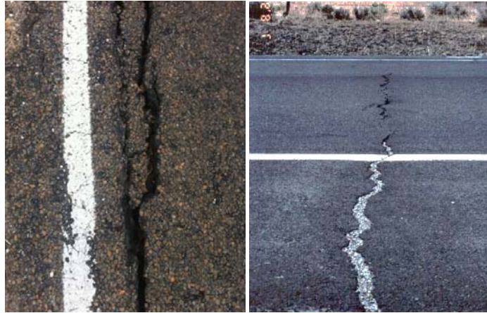
Figure 2. 4: Longitudinal (left) and transverse (right) cracking
