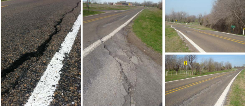
Figure 3. 2: Surficial pavement damages due to expansive subgrade soil
