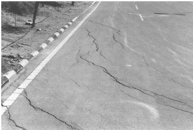
Figure 2-2 Flexible pavement failure (Al Rawas et al., 2005)
