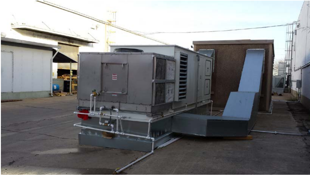
Figure 3-2 Modular Data Center: Shows Hot Data Center Return Duct
