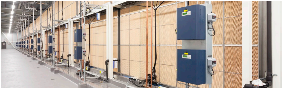
Figure 2-8 DEC media used at Facebook's data center at Luleå, Sweden [31]
