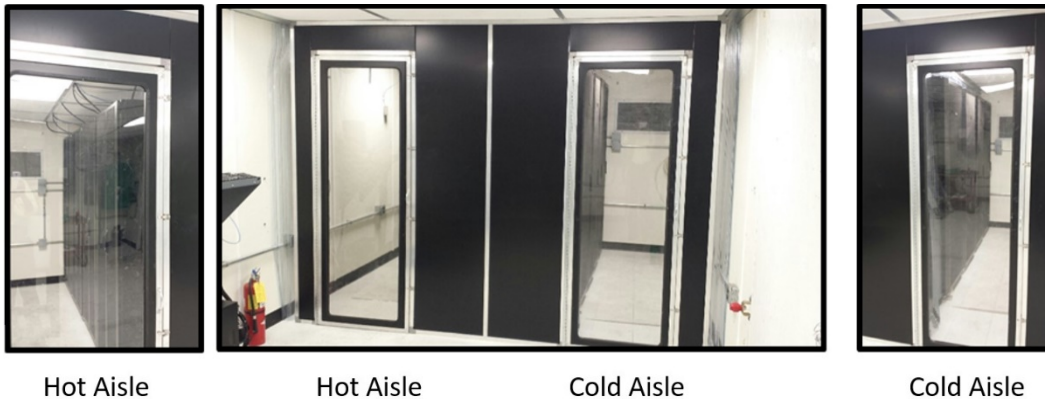
Figure 3-4 Hot/Cold aisle configuration inside the IT pod
