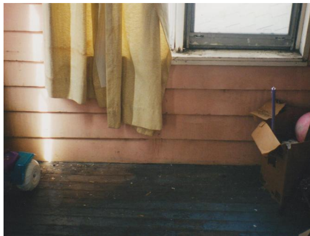
Figure 4-9 House O Poor Condition of Floor Paint
