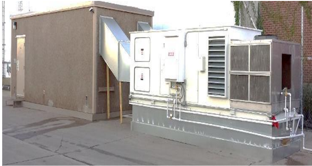
Figure 29 Data center facility
