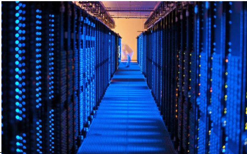
Figure 1 Amazon data center [1]
