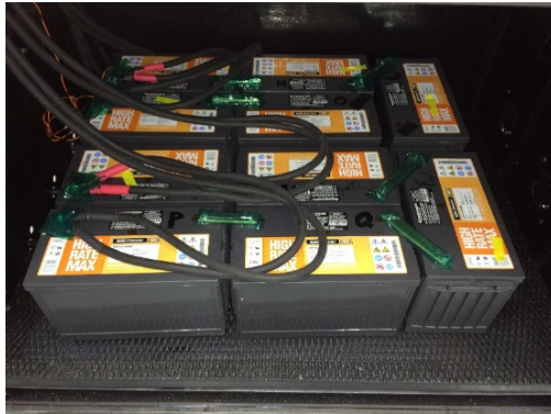
Figure 3-11. 5S/2P C&D UPS12-400MR battery assembled in a test chamber. Two sets of 3/0 wire is connected to each series set of cells.
