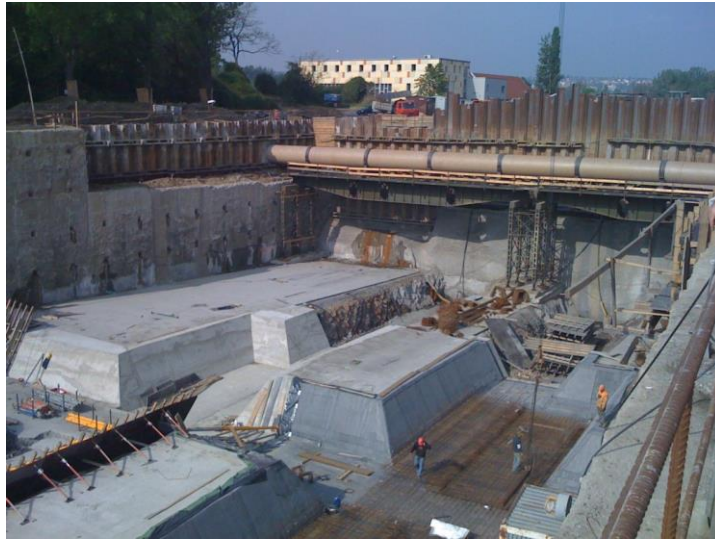
Figure 2-7 Blanka Tunnel in Prague, Czech Republic, a Section Constructed with Open-cut Method (Špačková, 2012)
